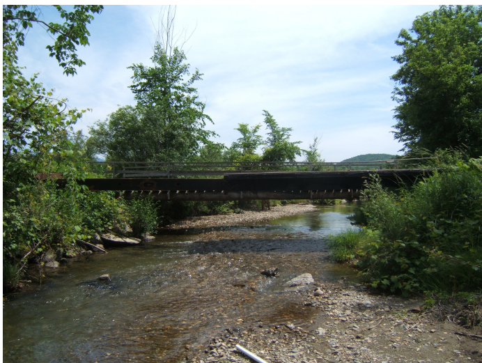
Figure bb. Recommended structure removal, steel bridge out of use upstream of Plains Road bridge
