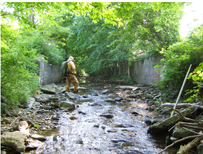
Figure ss. Old concrete abutment recommended for removal
