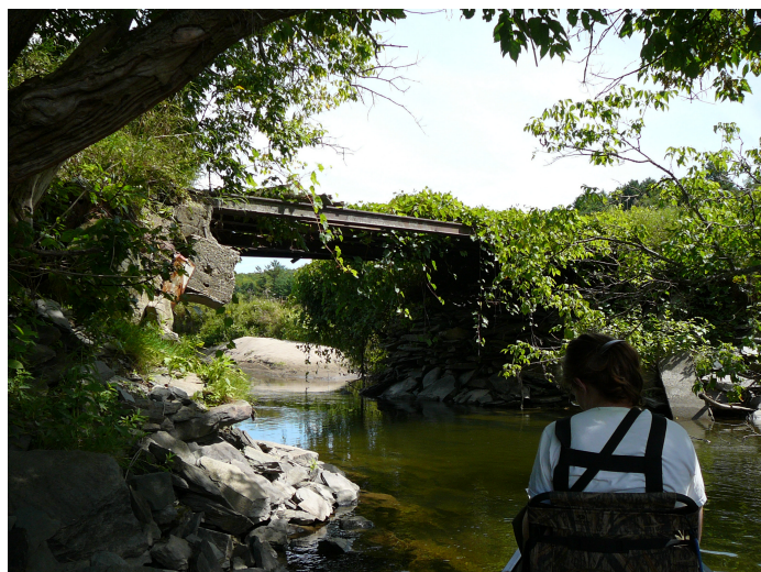
Figure p. Undermining abutments at structure downstream of junk car and Pettingill Road.
