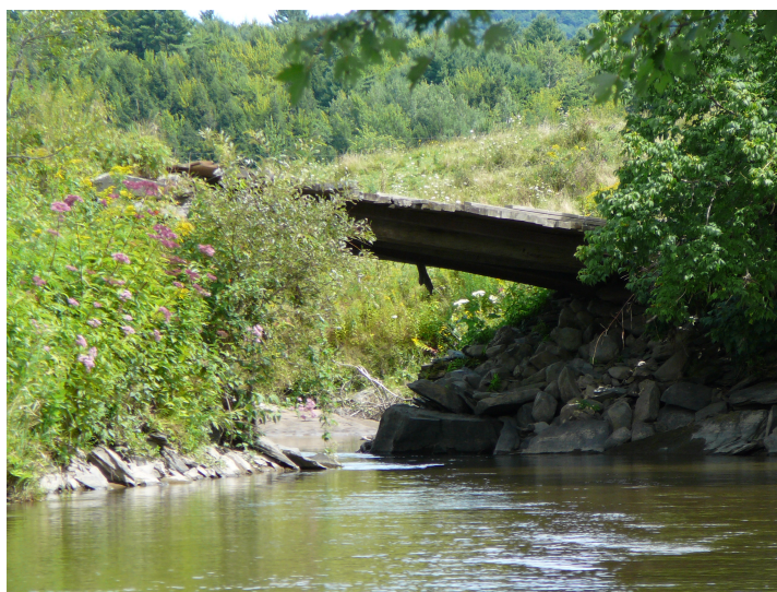
Figure m. Channel constriction, potential replacement project
