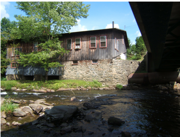
Figure u. Encroachment/hardbank downstream of Rte 15 dam
