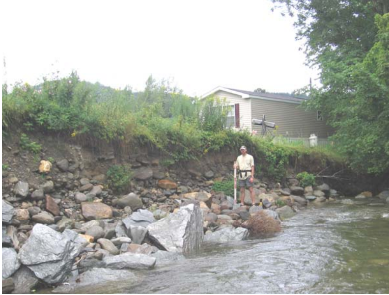
Figure 12: Failed Rip-Rap along T3-01B
