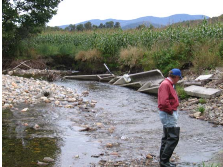
Figure 15: Bank failure and debris along T4-03
