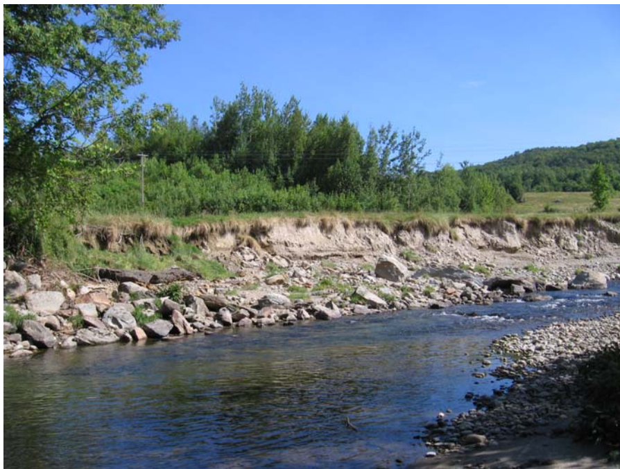
Figure 4: Failed Rip Rap just Downstream of Longley Bridge.
