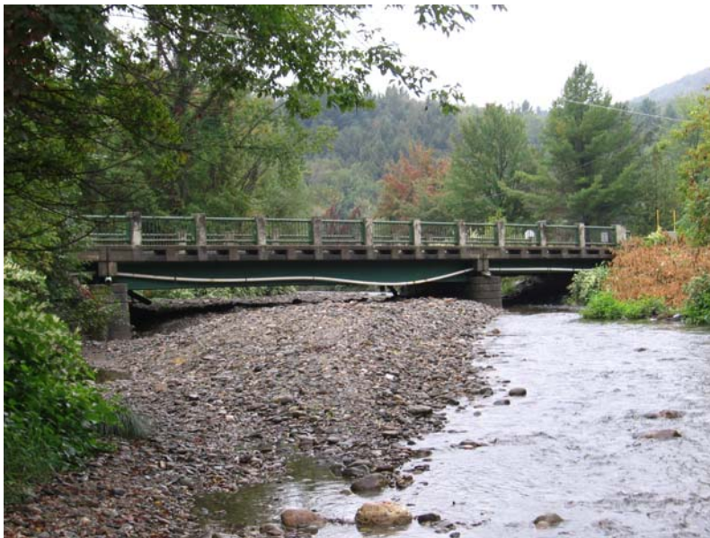
Figure 20: T2-01 Bridge Clogged with Sediment
