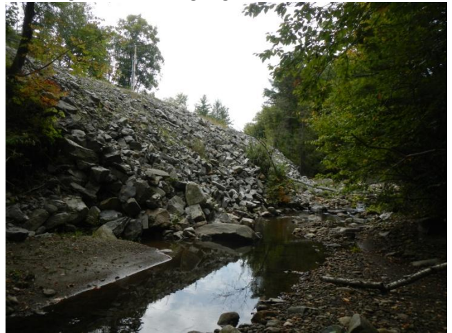
Figure 4.22: Extreme encroachment along Route 11 on reach T5.08.
