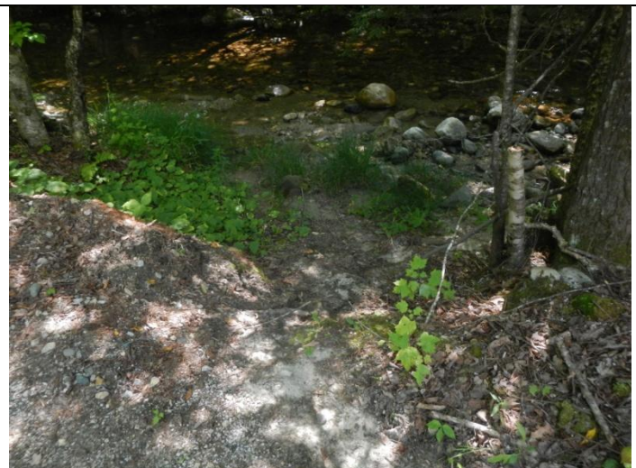
Smokeshire Rd. ditches add sediment in the river
