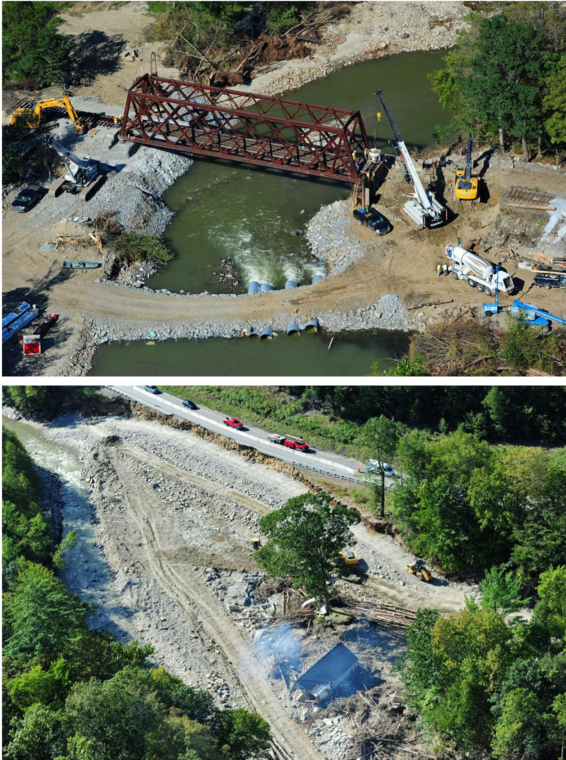
Figure 1.9: Major repairs to a railroad bridge on Reach M10 in Chester. Destroyed house, damage to Route 11, and extensive earth work along the Middle Branch (photos courtesy of Mansfield Heliflight).
