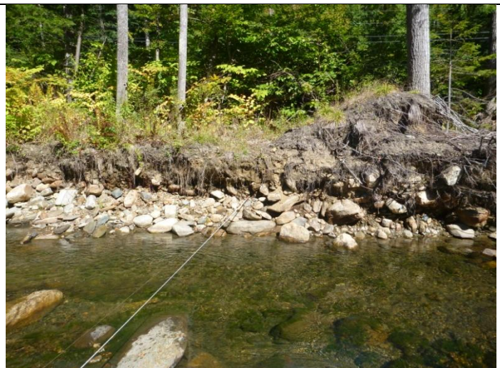
Upper cross-section left (north) unstable bank
