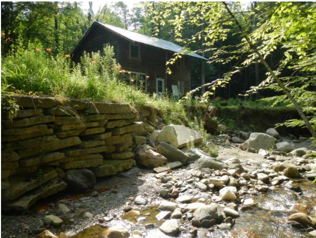
Figure 4.21: Encroachment from development along Potash Brook (T5.S3.a.01).
