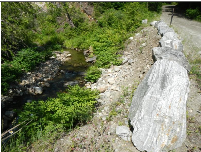
Actively eroding bank along Lamson Rd.
