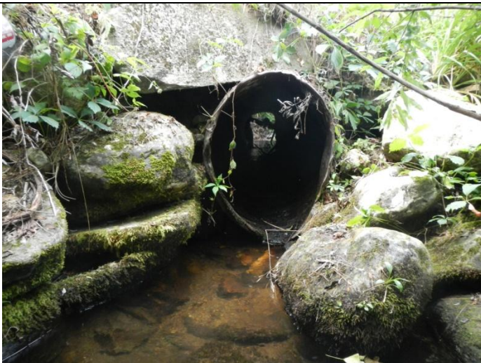
Outlet of severely undersized culvert under farm road
