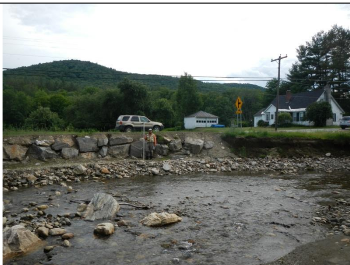
Raw bank erosion and armor along Rt-11
