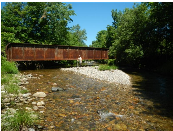
Railroad bridge with low capacity due to aggradation
