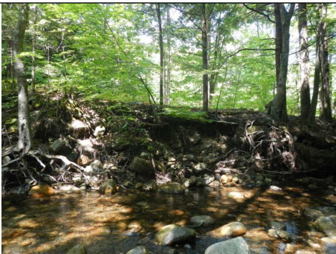
Bank scour and evidence of widening
