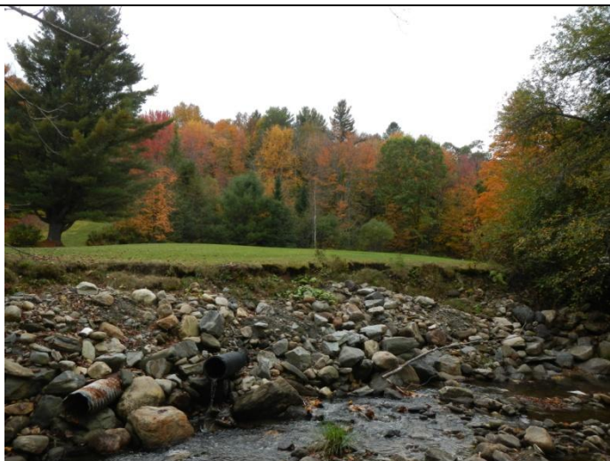
T.S. Irene scour and widening
