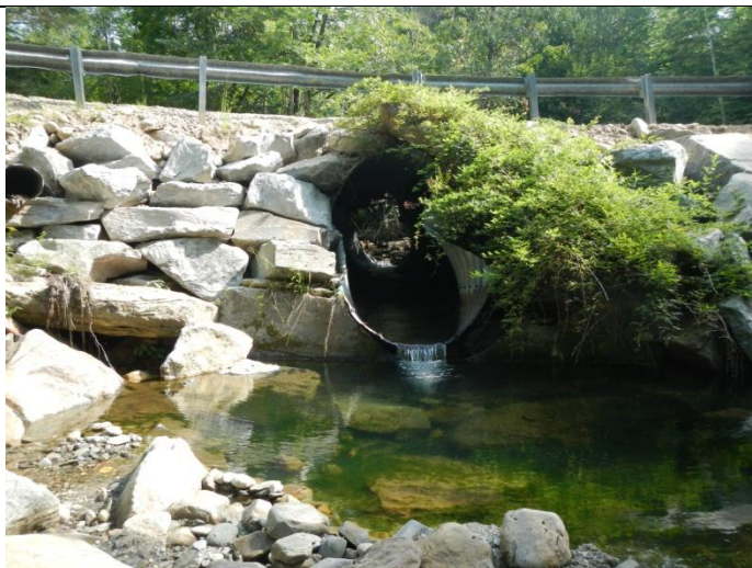
Culvert needing replacement along Potash Brook Rd.
