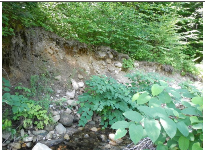
Scoured banks depict recent widening by the channel
