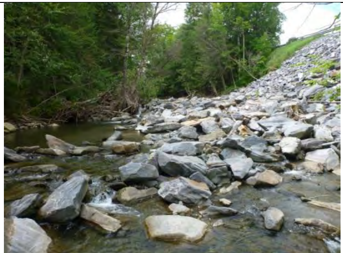
Two bed and bank armoring sites were observed at damage sites along North Danville Rd
