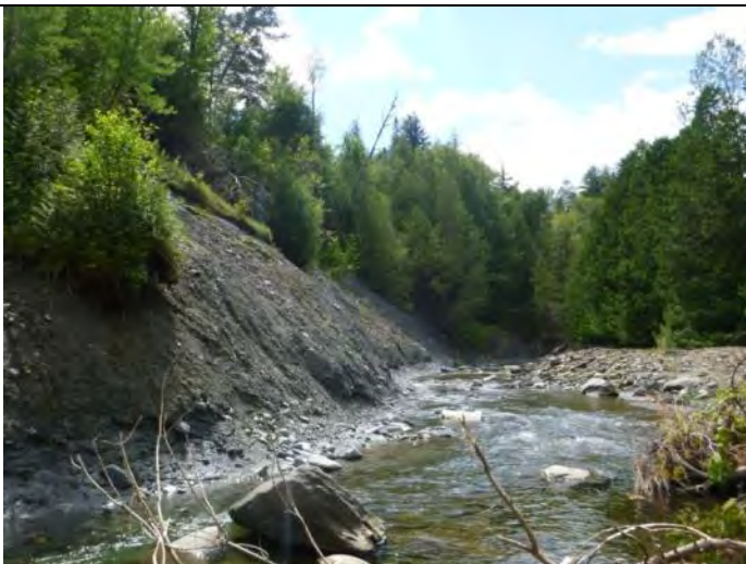
Numerous large mass failures were observed along the right bank
