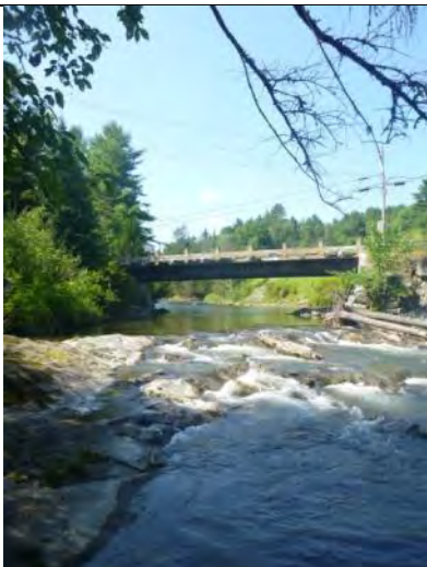
Mid-reach looking upstream - stable rocky banks and the undersized TH-8 bridge in disrepair
