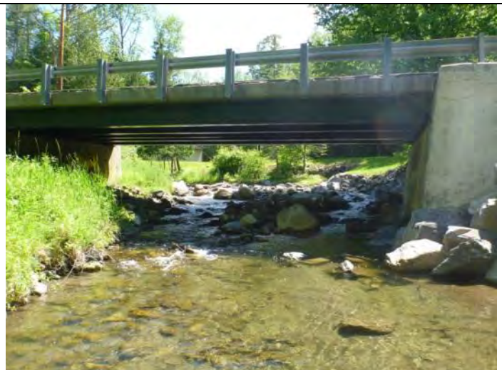
Coarse deposition upstream of undersized Red Village Road bridge
