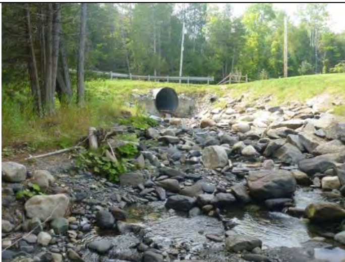
Perched culvert and recent bank erosion, armoring, and channel degradation below Cormier Rd
