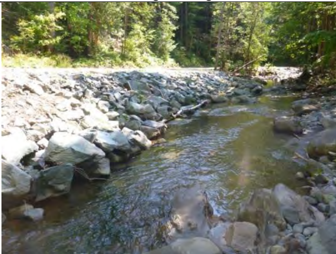
Encroachment and armoring along Water Andric Rd
