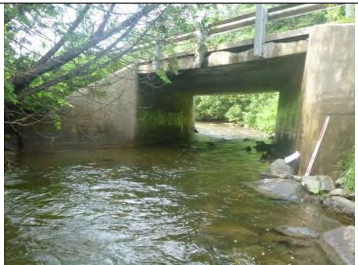
Undersized bridge at South Wheelock Road
