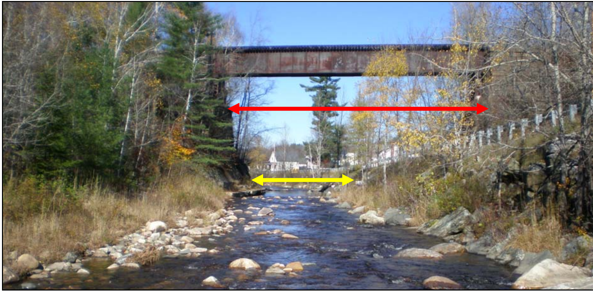
Figure 1: The railroad bridge span on M11-A is adequate for the Mill River (red line), however, location of Route 155 in relation to the bridge and the river creates a channel constriction between the bridge abutment and the road (yellow line).
