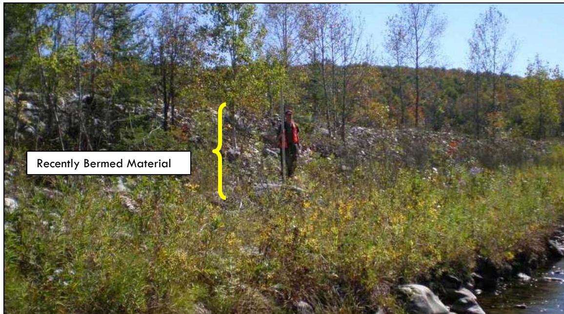
Figure 15. M07 has seen significant berming on the right bank causing a significant loss of floodplain access.
