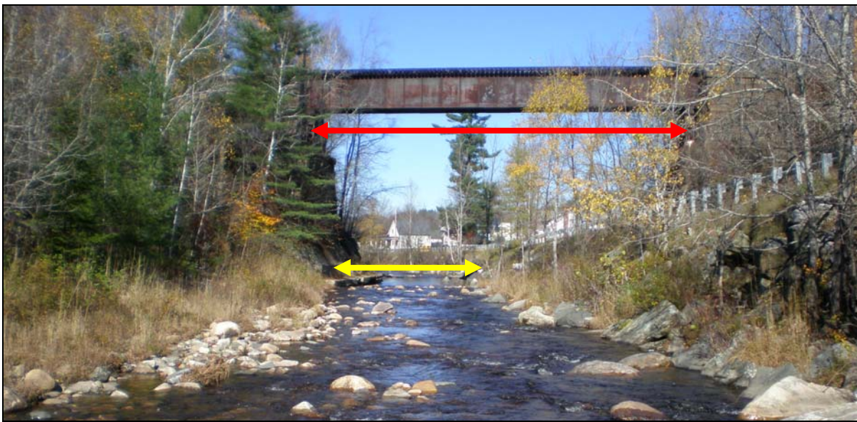
Figure 11: The railroad bridge span on M11-A is adequate for the Mill River (red line), however, location of Route 155 in relation to the bridge and the river creates a channel constriction between the bridge abutment and the road (yellow line).
