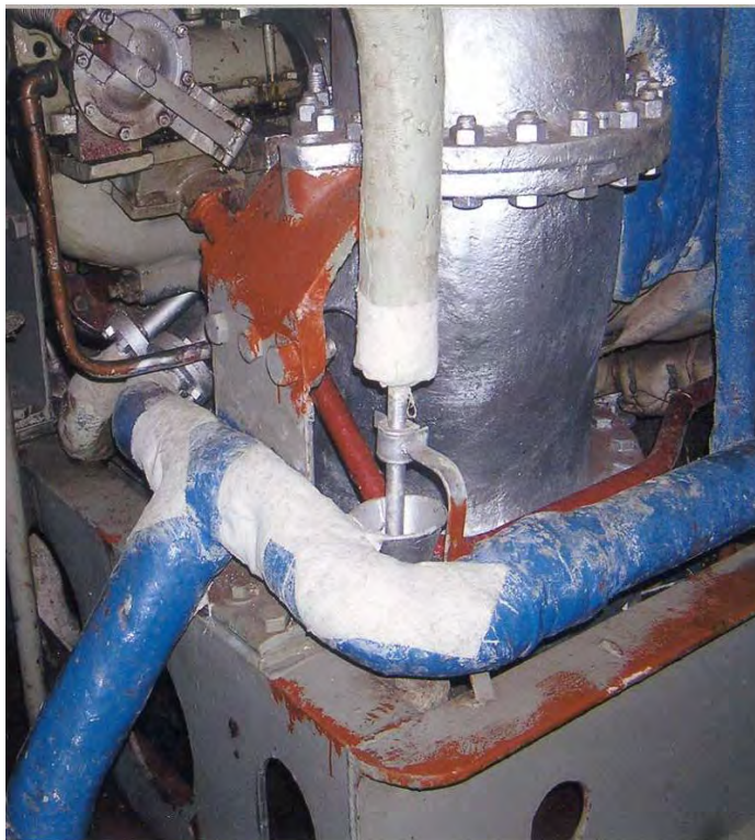
Photo courtesy of Laura S. Johnson Patched asbestos pipe wrapping on the ex-USS Oriskany.
