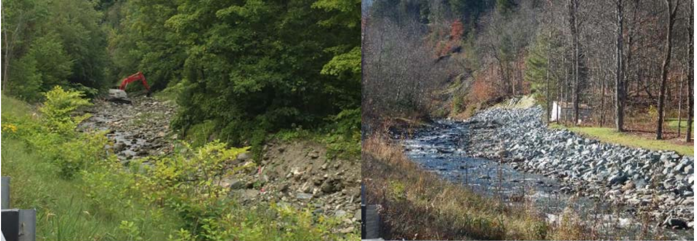
Photo 6 – Before (Left) and after (Right) stream bank alteration work along Locust Creek along the historic sampling reach in 2017.
