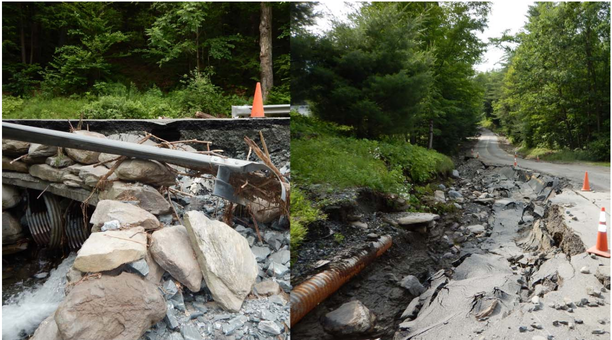
Photo 2 – Flood damage that occurred on July 2, 2017 along Podunk Brook in W. Hartford.
