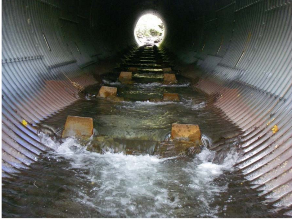
Photo 11– Mill Brook baffles used to replace the original 1995 baffles, following TS Irene. These baffles failed in 2013
