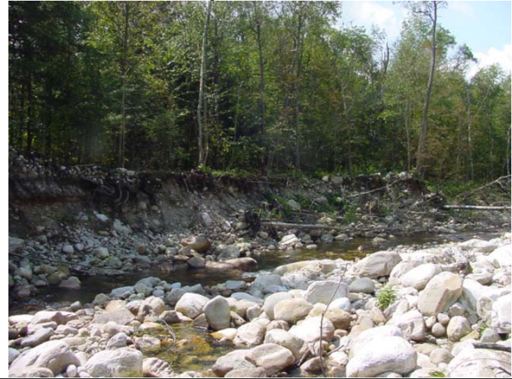
Reach/Segment: M06T3.02 Photo No.: DSC00047.JPG Date: 9/7/2006 View/Description: LB Erosion
