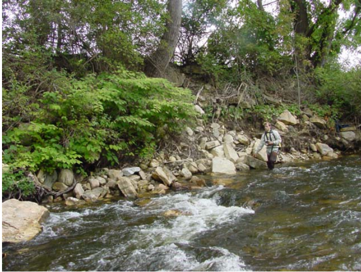
Reach/Segment: M06b Photo No.: DSC00028.JPG Date: 9/20/2006 View/Description: RB Erosion / Revetment
