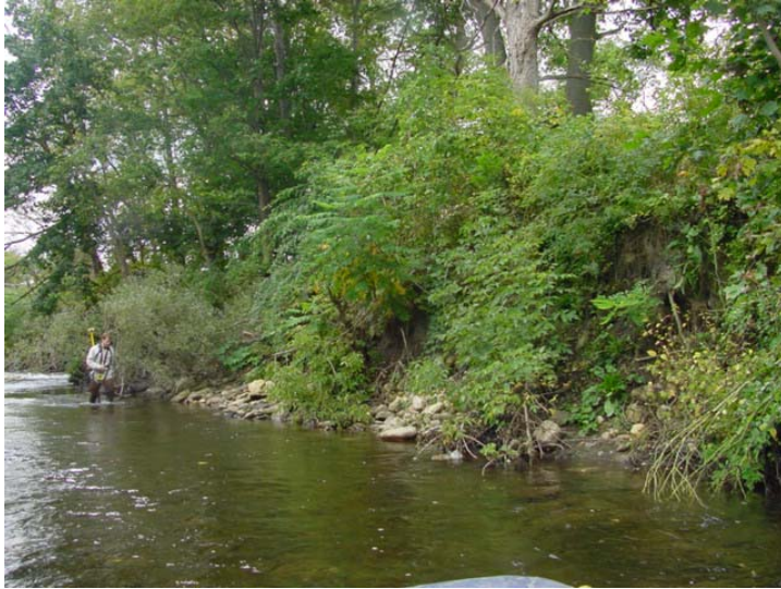
Reach/Segment: M06b Photo No.: DSC00024.JPG Date: 9/20/2006 View/Description: U/S Erosion on LB
