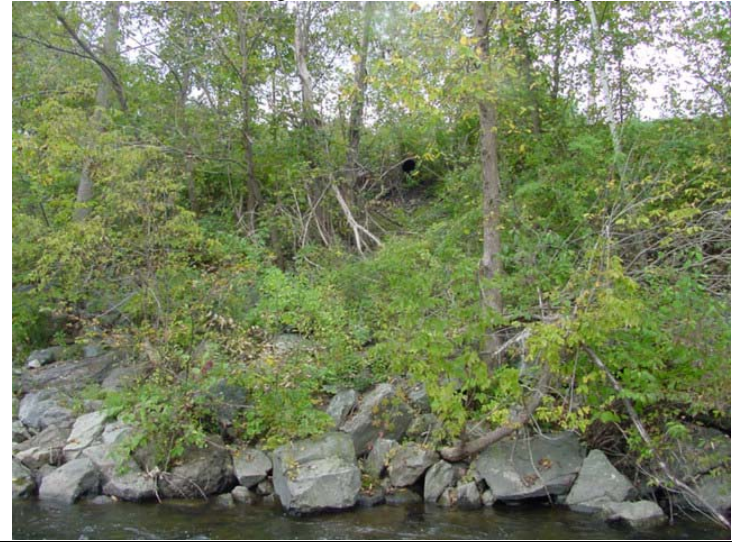
Reach/Segment: M06a Photo No.: DSC00037.JPG Date: 9/20/2006 View/Description: LB Outfall pipe
