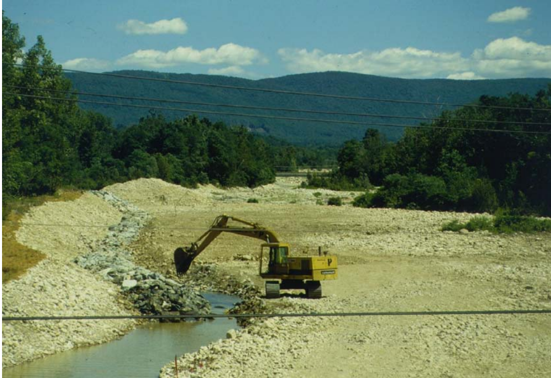
Plate 3: Roaring Branch Streambank Armoring Following 1987 Flood.
