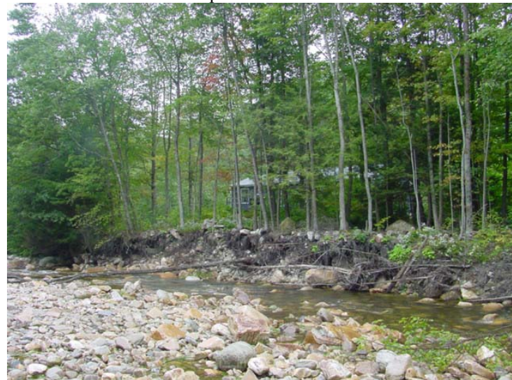
Reach/Segment: M06T3.04 Photo No.: DSC00015.JPG Date: 9/5/2006 View/Description: RB Erosion
