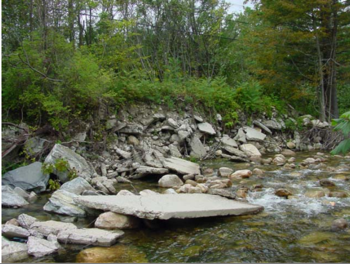
Reach/Segment: M06T3.03 Photo No.: DSC00031.JPG Date: 9/6/2006 View/Description: RB Erosion – old abutments
