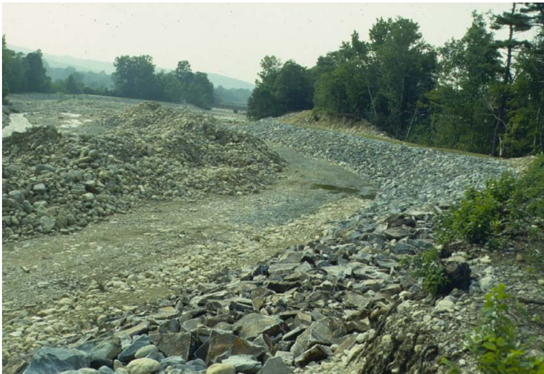
Plate 4: Roaring Branch, Reconstruction of Failed Berm Following 1987 Flood.
