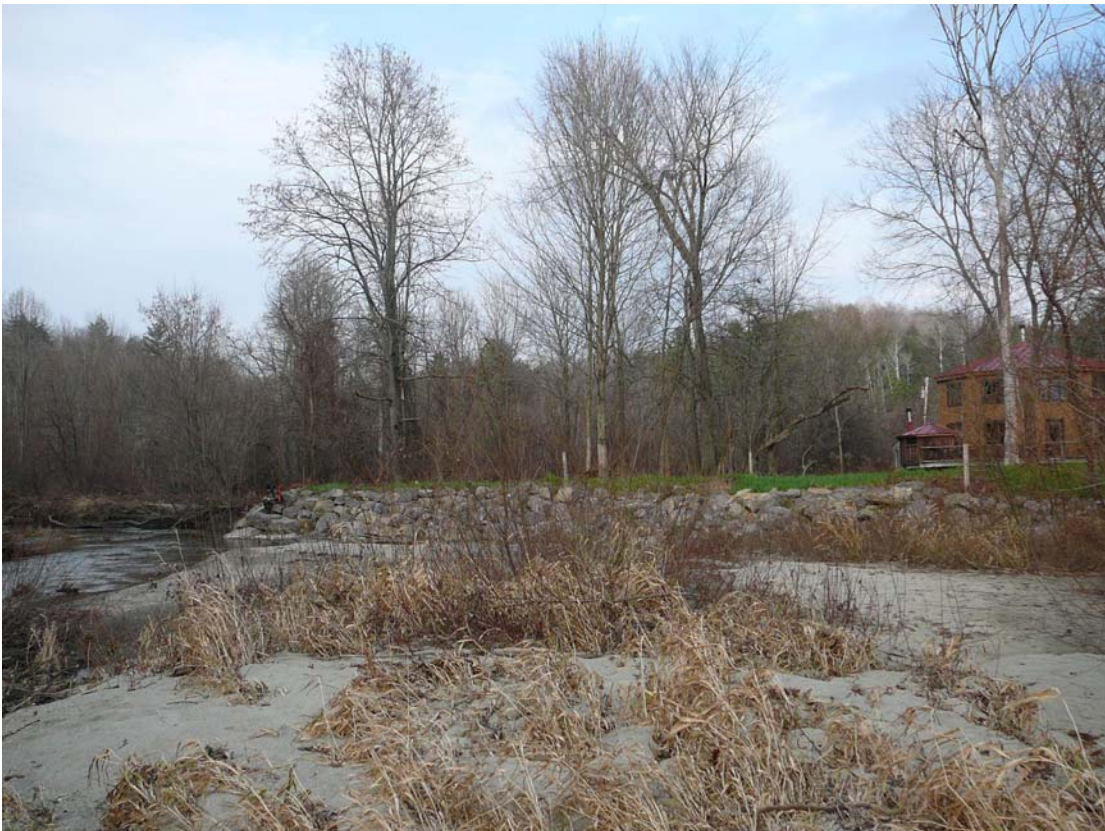
Figure 2. Rip-rap armoring installed circa 2006 along right bank at Dexter Lorange property off Lewis Creek Road in Hinesburg (Segment M15-A). View downstream, 29 November 2006.
