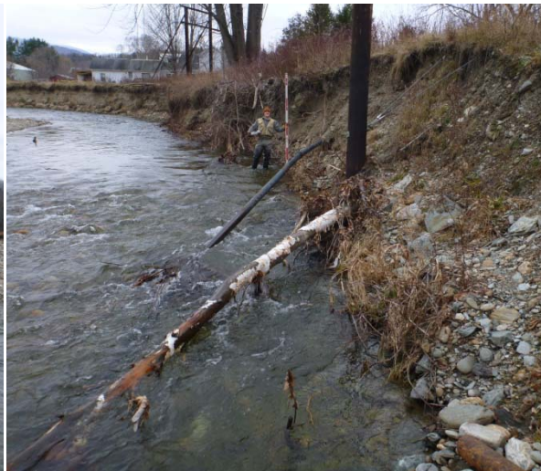
Figure 21: 400 feet of bank erosion upstream of VT Rte. 15
