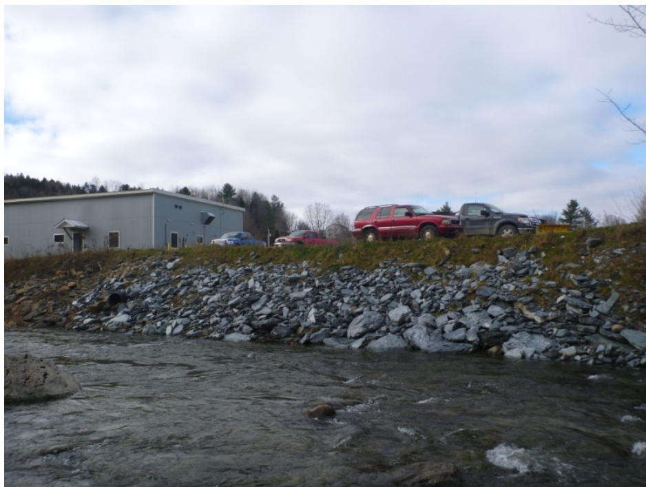
Figure 12: Bank armoring in Reach M01
