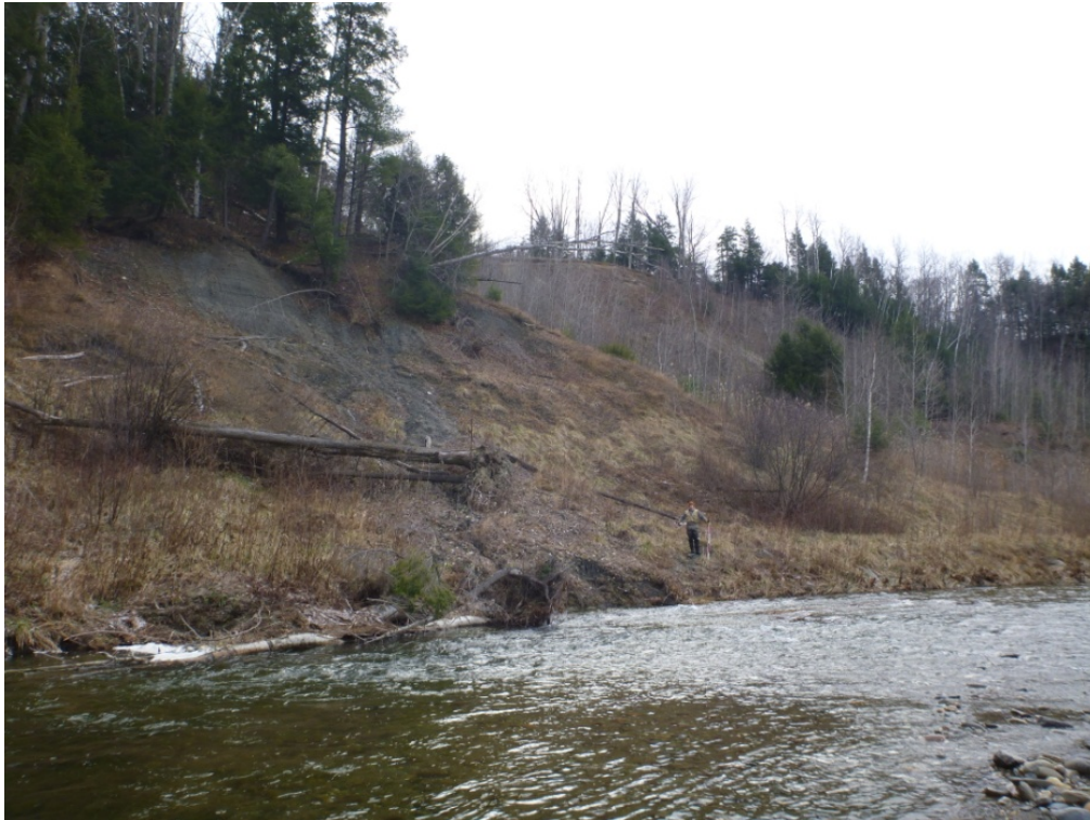
Figure 22: A 180' by 70' Mass failure on the right bank. The largest mass failure (350' by 150') is in the background approximately 100' from the channel
