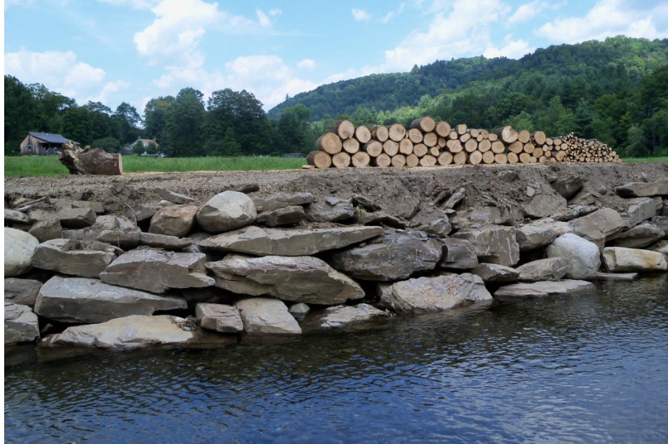
Figure 4.16 Newly installed riprap with trees cut along the bank in segment R19-B
