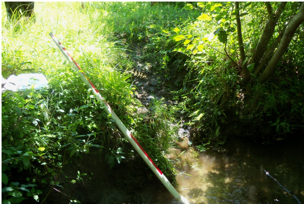
Figure 4.32 Animal crossing and eroded bank
