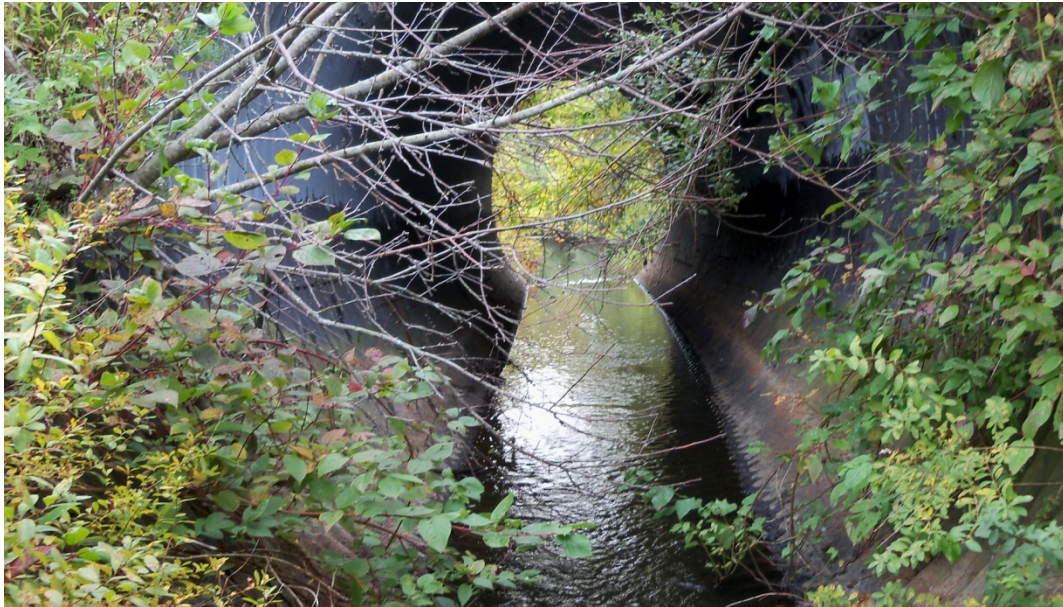
Figure 4.77. Reduced aquatic organism passage and geomorphic incompatibility at Middle Brook Road Culvert
