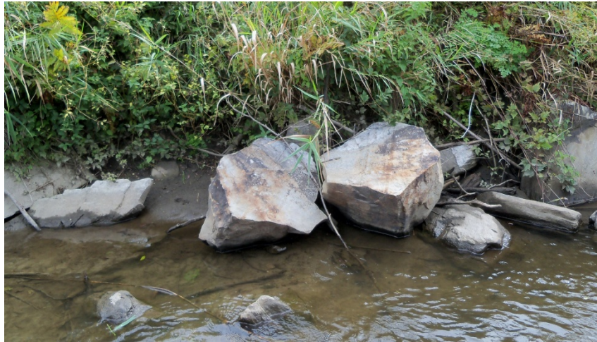
Figure 4.61 Outflanked riprap in R16T2.03S1.02-B
