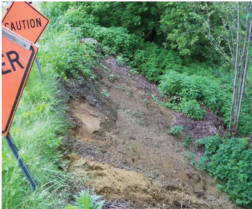
Figure 7.23. Mass Failure (unstable valley wall of the Neshobe River) located adjacent to Wheeler Rd (BCE, 5/25/2011)
