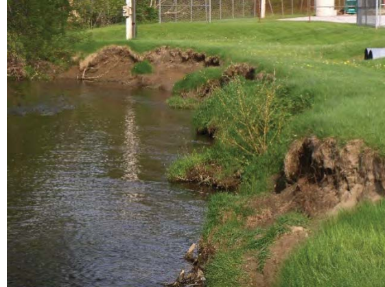
Figure 7.3. Lack of buffer and bank erosion in the vicinity of the wastewater treatment plant (BCE, 5/7/2010)
