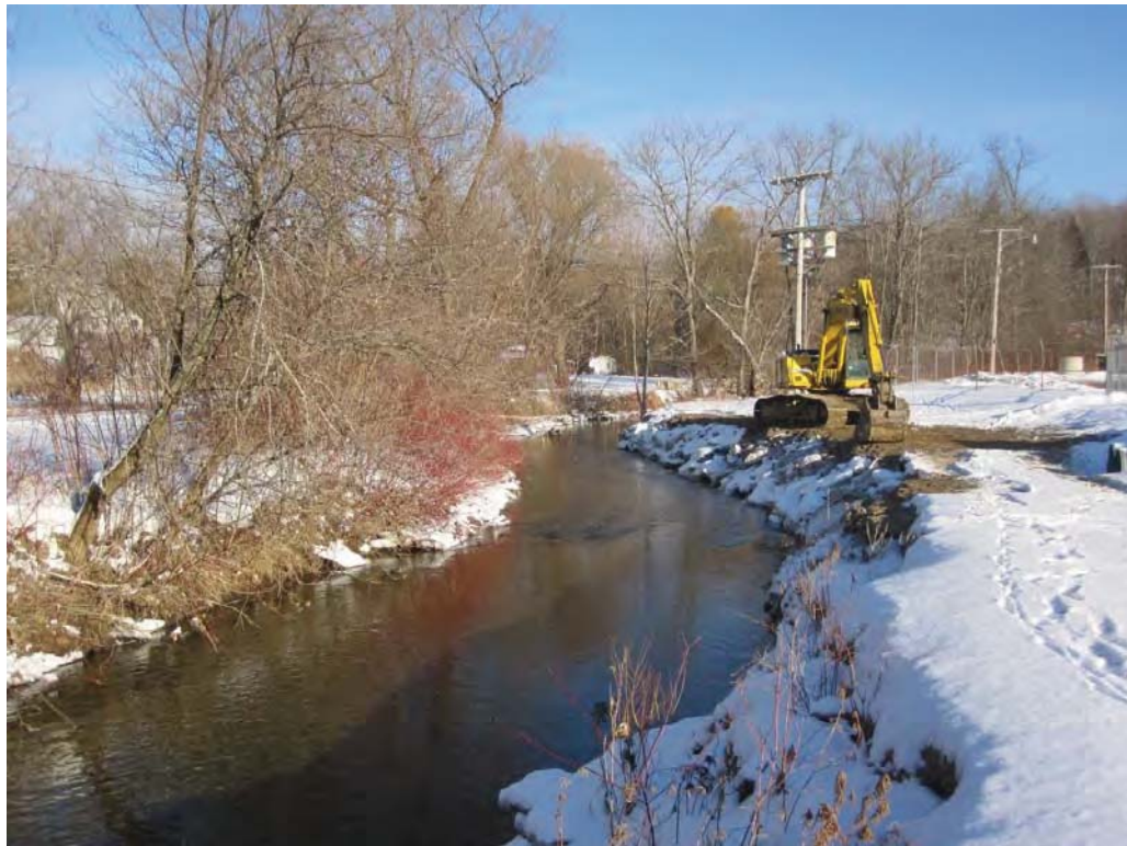
Figure 7.20. Newly riprapped section of Neshobe River adjacent to WWTF (Photo by Ethan Swift)
