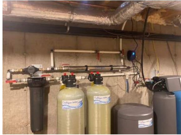
Photo #8 : View of 583 Quarry Hill Road POET system.
