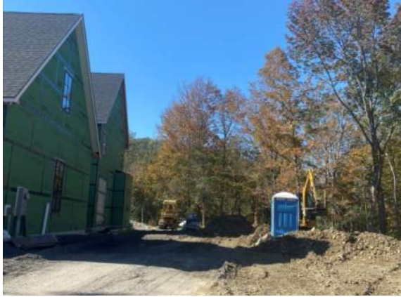
Photo #1 : View of northern side of the 583 Quarry Hill Road residence, facing west. TP-1 is located north of the building.
