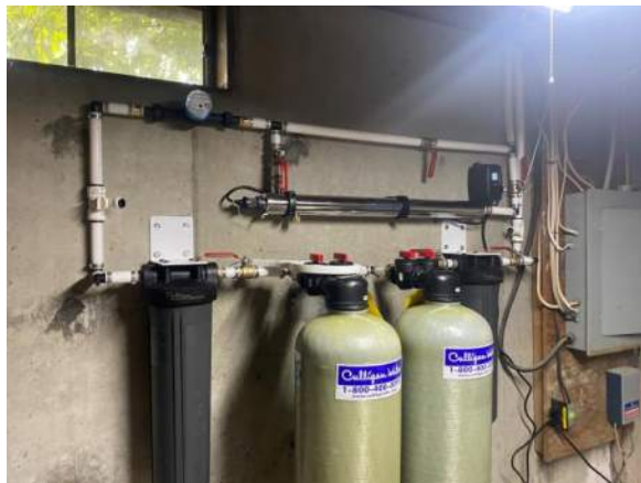
Photo #9 : 871 North Pownal Road POET system.
