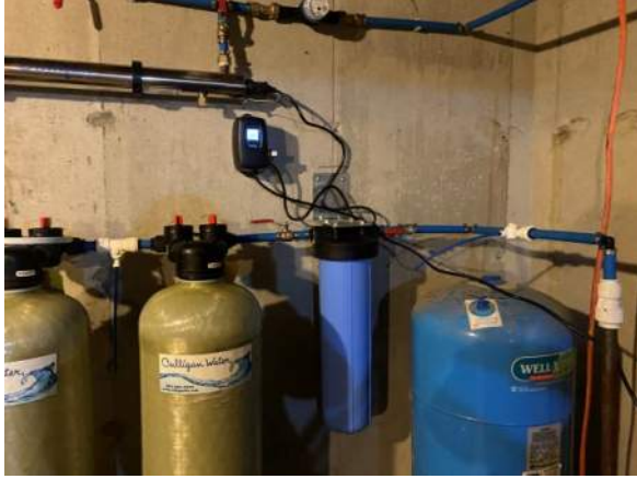
Photo #7 : View of 581 Quarry Hill Road Point of Entry Treatment (POET) system.
