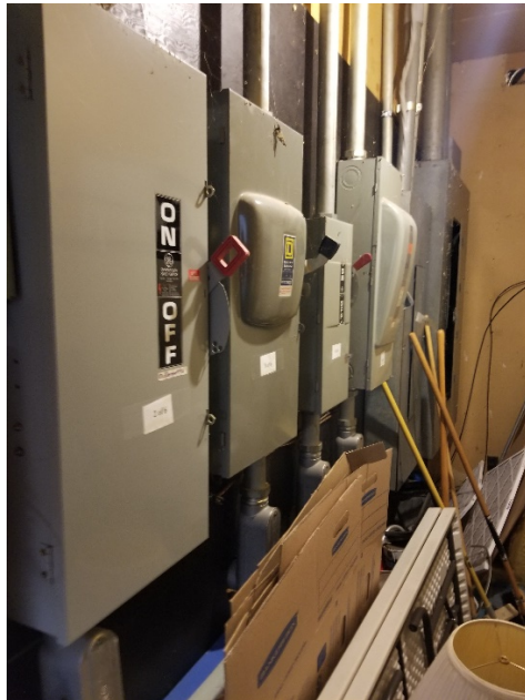
Plate 12. Utility room in Adult Learning Center with electrical power switches.
