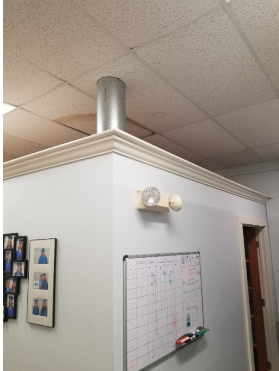
Plate 11. Heating duct work, Adult Learning Center. Note water damage in ceiling tile.
