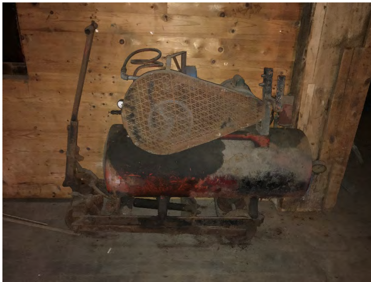
Photograph 20: Oil-stained air compressor on the first floor of the former grain elevator and storage building.
