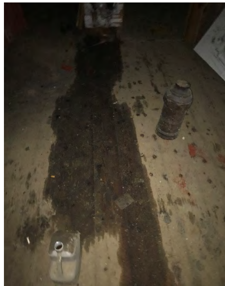
Photograph 24: Staining on the wooden floor in the maintenance room in the eastern portion of the second floor of former grain elevator and storage building.
