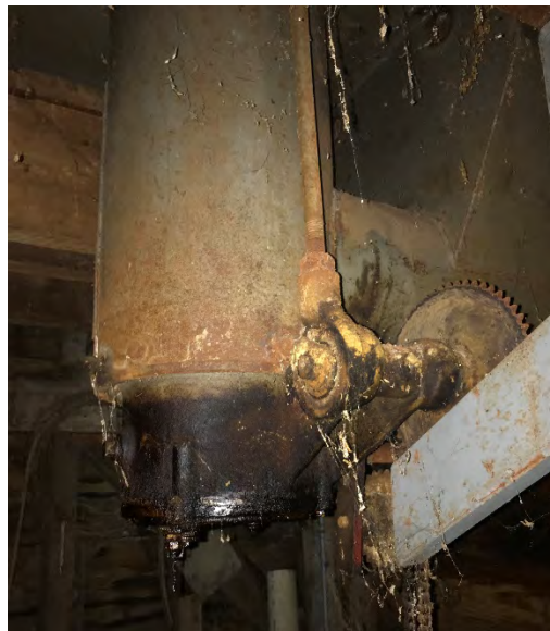
Photograph 28: Oily components typical of infrastructure located throughout the former grain elevator and storage building.
