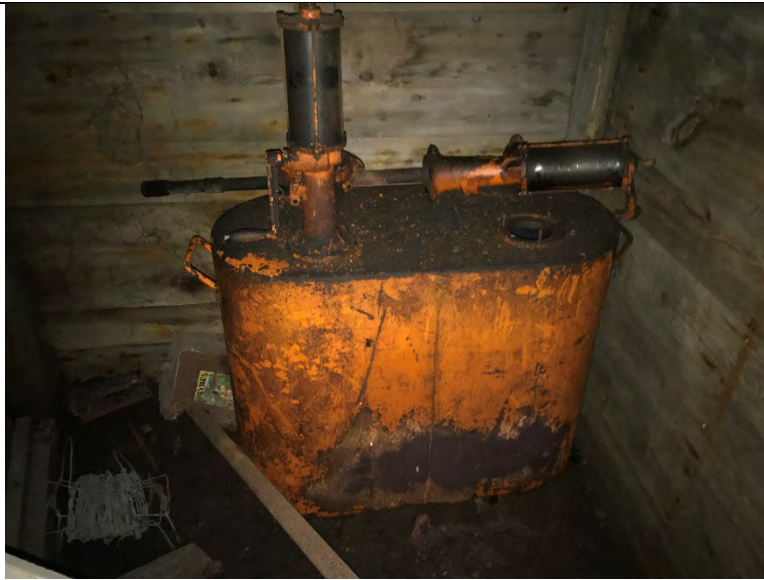
Photograph 23: Portable fuel tank located in the northwestern portion of the first floor of former grain elevator and storage building. An unidentified liquid was observed through the fill port of the tank.
