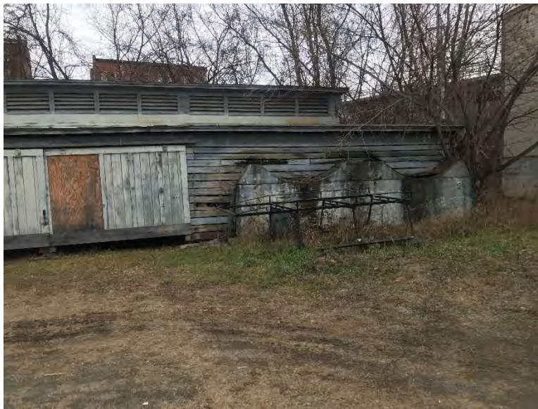
Photograph 4: Eastern façade of the carriage barn building, looking west. Two, semi-circular above ground storage tank cradles are shown on the right.
