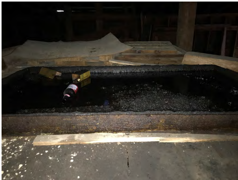
Photograph 30: Oily pan on an elevated wooden platform beneath the elevator's pulley system.
