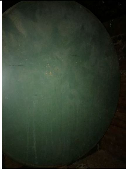
Photograph 25: Western side of the molasses storage tank on the second floor of former grain elevator and storage building.
