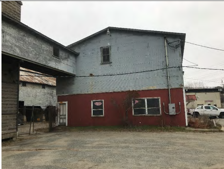
Photograph 5: Southern façade of the former retail and storage building, looking north. The elevated catwalk connecting the building to the former grain storage building is pictured, as well as the coal hoppers shed in the background on left.
