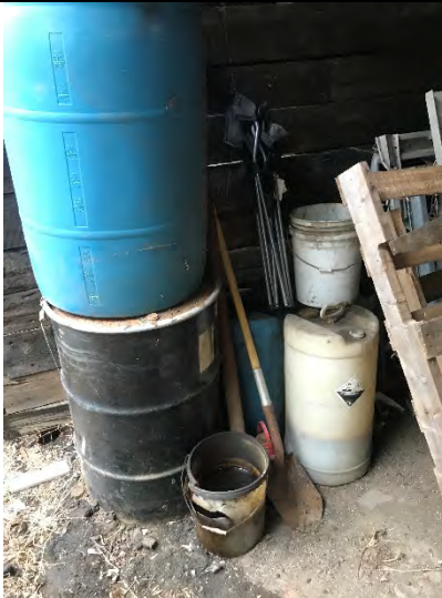
Photograph 17: Drum storage and oil staining in the northernmost bay of the coal hoppers shed.
