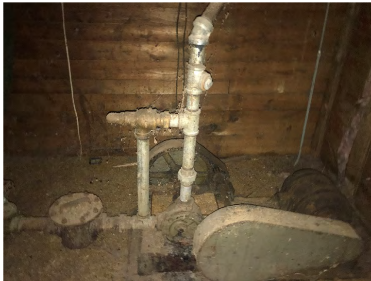
Photograph 26: Pump connected to the molasses storage tank on the second floor of the former grain elevator and storage building.
