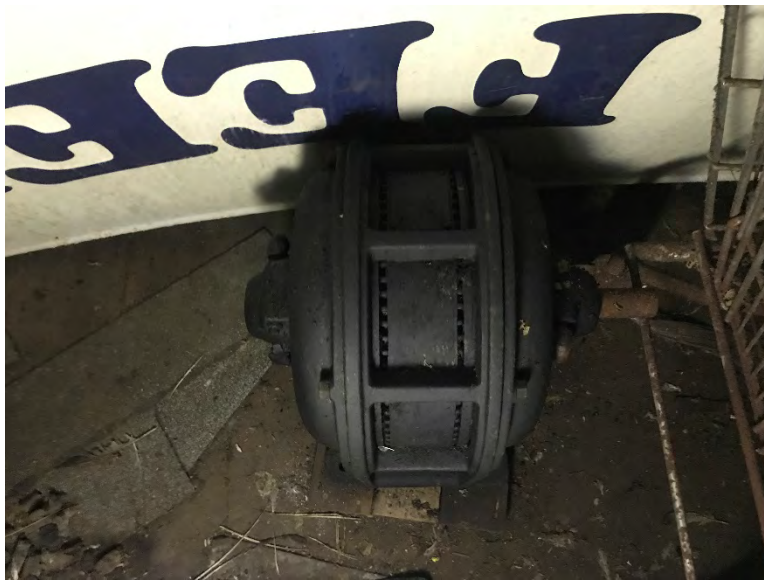
Photograph 22: Oil-coated motor in the southwestern portion of the first floor of former grain elevator and storage building.
