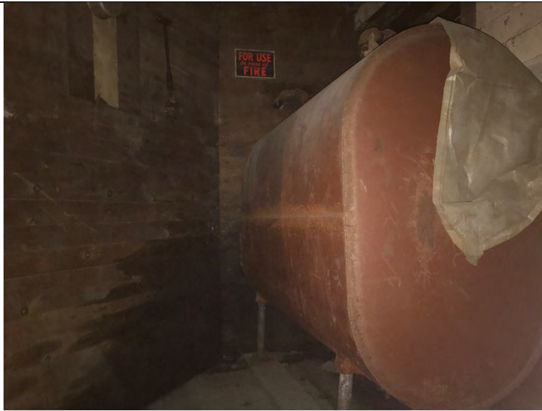
Photograph 19: 275-gallon fuel oil AST located in the northeastern portion of the former grain elevator and storage building.
