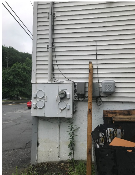
Photograph #16: Dumpster storage area and electrical panel to service building, located on southern side of building, looking north.
