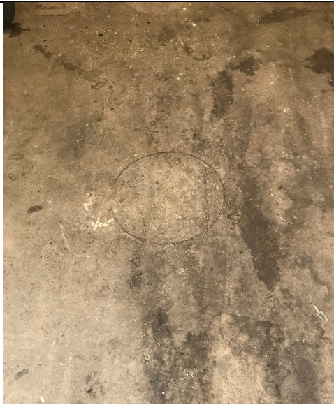
Photograph #13: Possible floor drain filled in with concrete located in single bay garage in southern portion of building.
