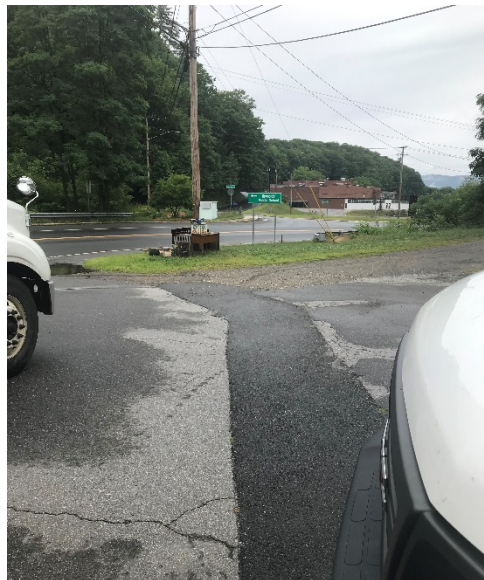
Photograph #4: Buried sewer line in cut-out of pavement, looking northwest toward Chester Road.
