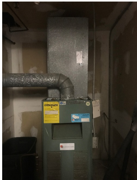
Photograph #8: Typical propane force hot air furnace, four units are in the building.
