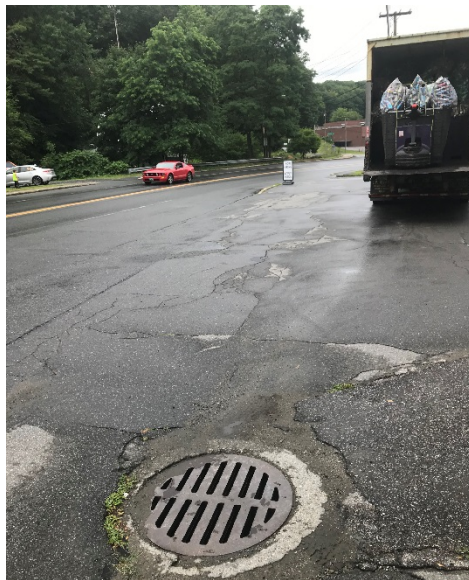
Photograph #14: Stormwater drain located in parking lot, accessed from Chester Road on western side of building, looking north.
