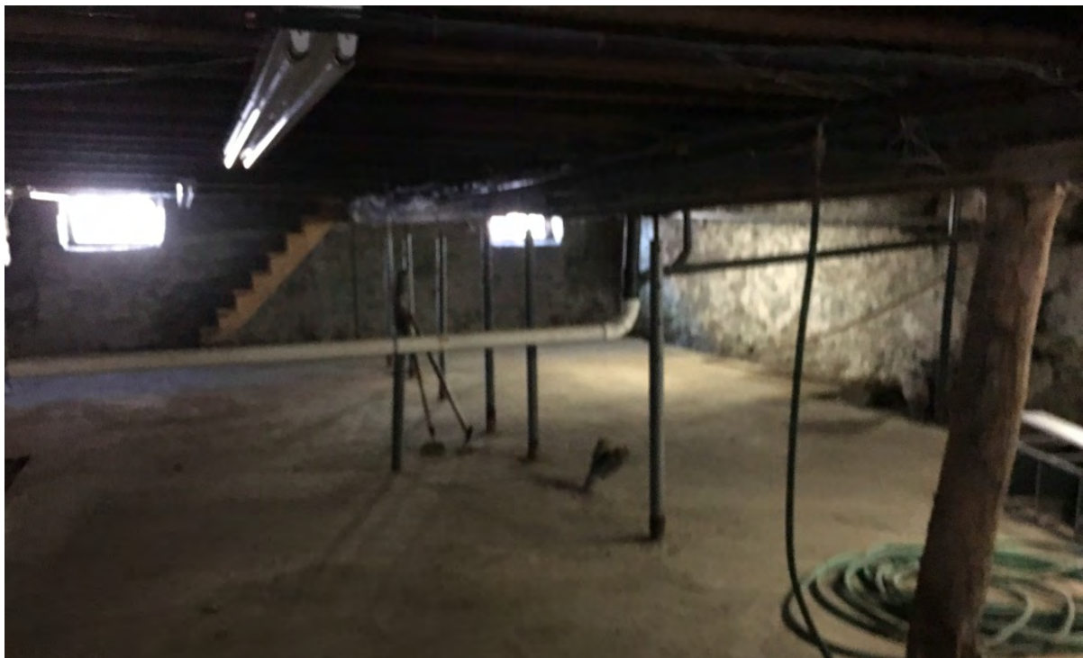
Photo 56: 15-17 Stebbins Street: Basement of the law office. Photo taken facing west by Sanborn Head on January 11, 2017.
