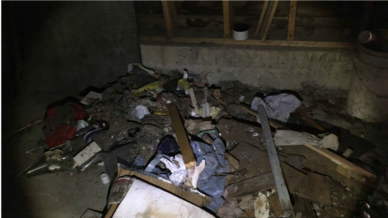
Photo 9: 14 Stebbins Street: Various construction and demolition debris was observed within the warehouse. Photo taken by Sanborn Head on January 10, 2017.
