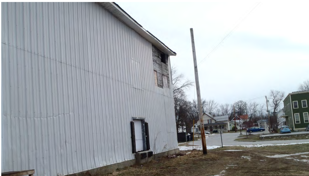
Photo 16: 14 Stebbins Street: The western side of the warehouse building. Photo taken facing south by Sanborn Head on January 10, 2017.
