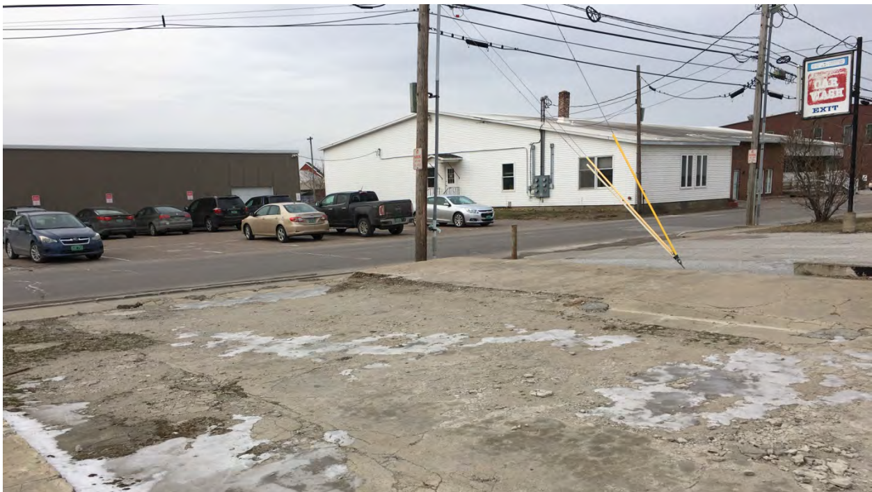
Photo 28: 25 Stebbins Street: The foundation of the building formerly located on 25 Stebbins Street; building was reportedly destroyed in a fire in 2006. Photo taken facing northeast by Sanborn Head on January 10, 2017.
