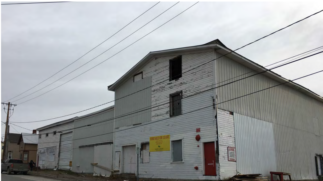
Photo 8: 14 Stebbins Street: The exterior of the warehouse building located at 14 Stebbins Street. Photo taken facing south by Sanborn Head on January 10, 2017.
