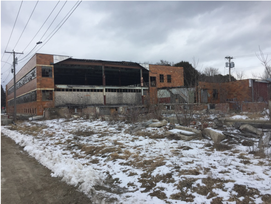
Photo 5: The Site looking northeast. Construction debris from the demolished building, two utility poles both with pole-mounted transformers, and the rear of the existing building can be seen.
