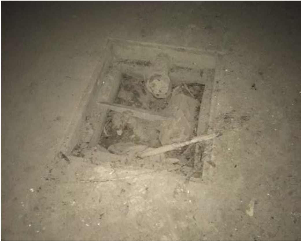
Photo 30: One of the pits observed in the basement.
