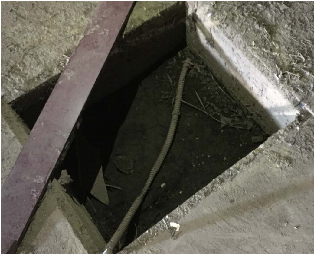
Photo 27: One of the pits observed in the basement.
