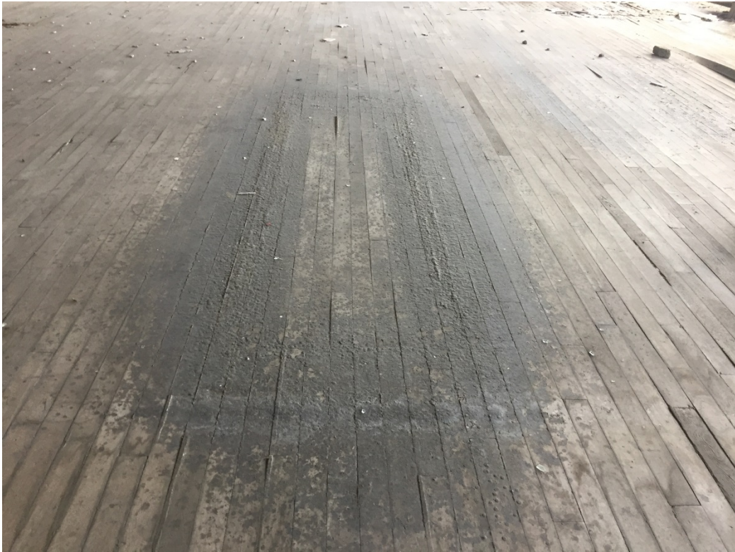
Photo 19: Staining, that appeared to be oily in nature, on the top floor of the building.
