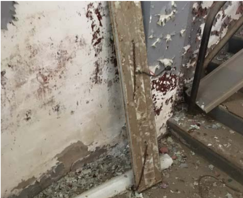
Photo 16: Peeling paint and an inactive tube fluorescent light in the stairwell.
