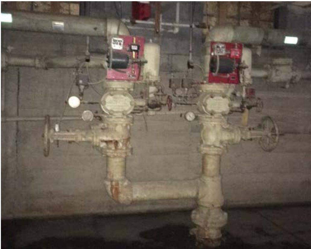
Photo 32: The sprinkler distribution system in the basement.
