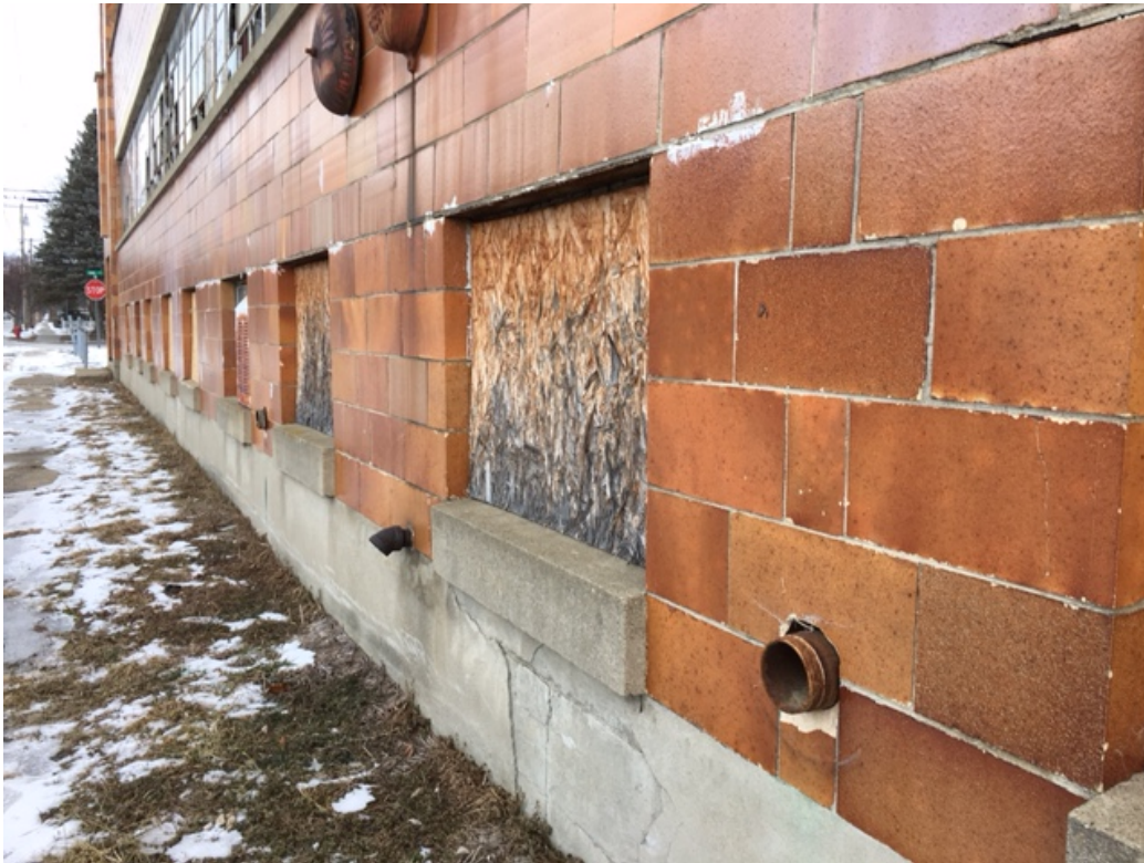
Photo 12: Three pipes, which may be related to the sprinkler system, on the west wall of the building.
