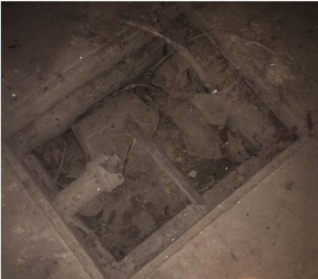
Photo 26: One of the pits observed in the basement.
