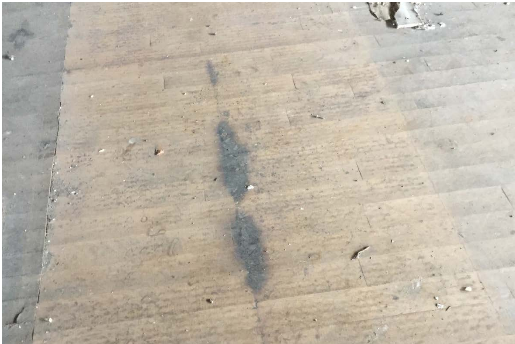
Photo 20: Staining, that appears to be oily in nature, on the top floor of the building.
