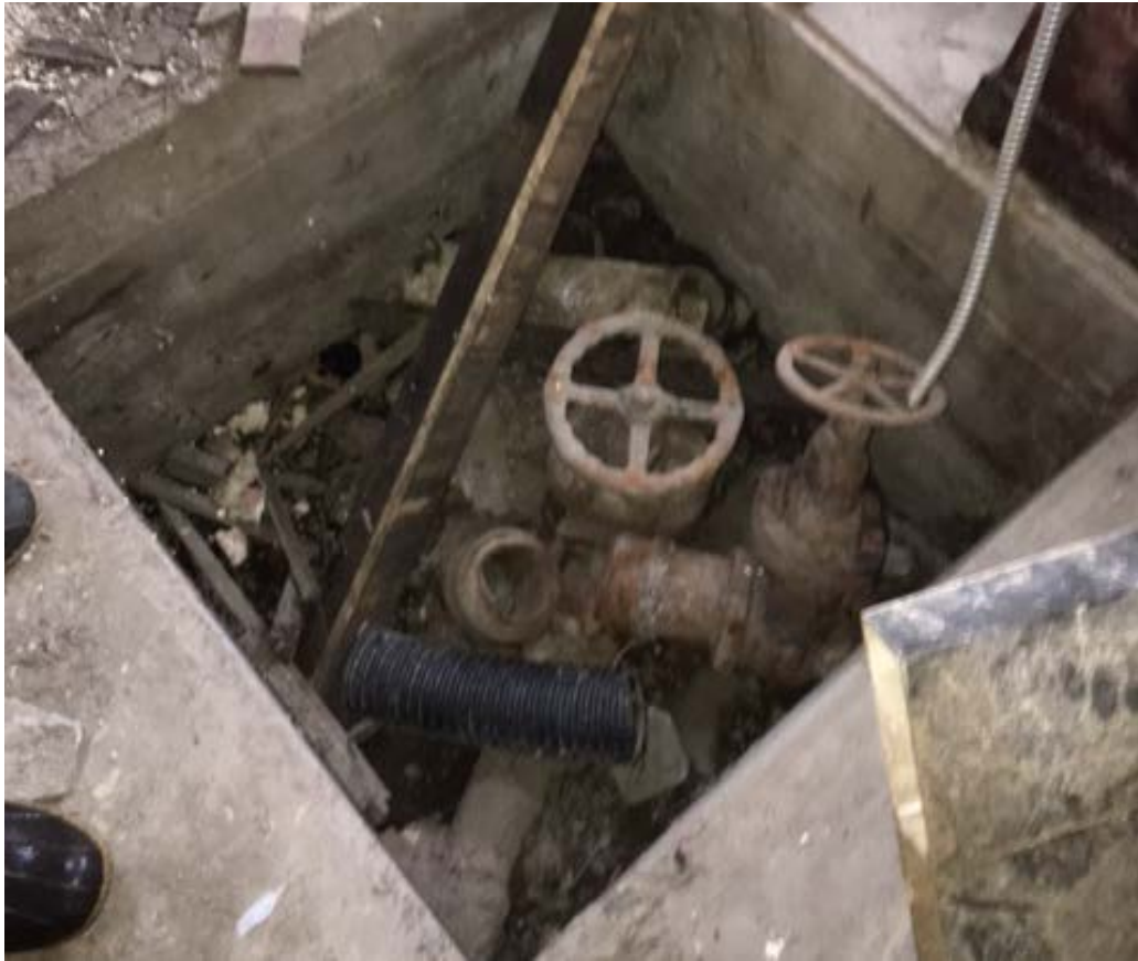
Photo 31: One of the pits observed in the basement.
