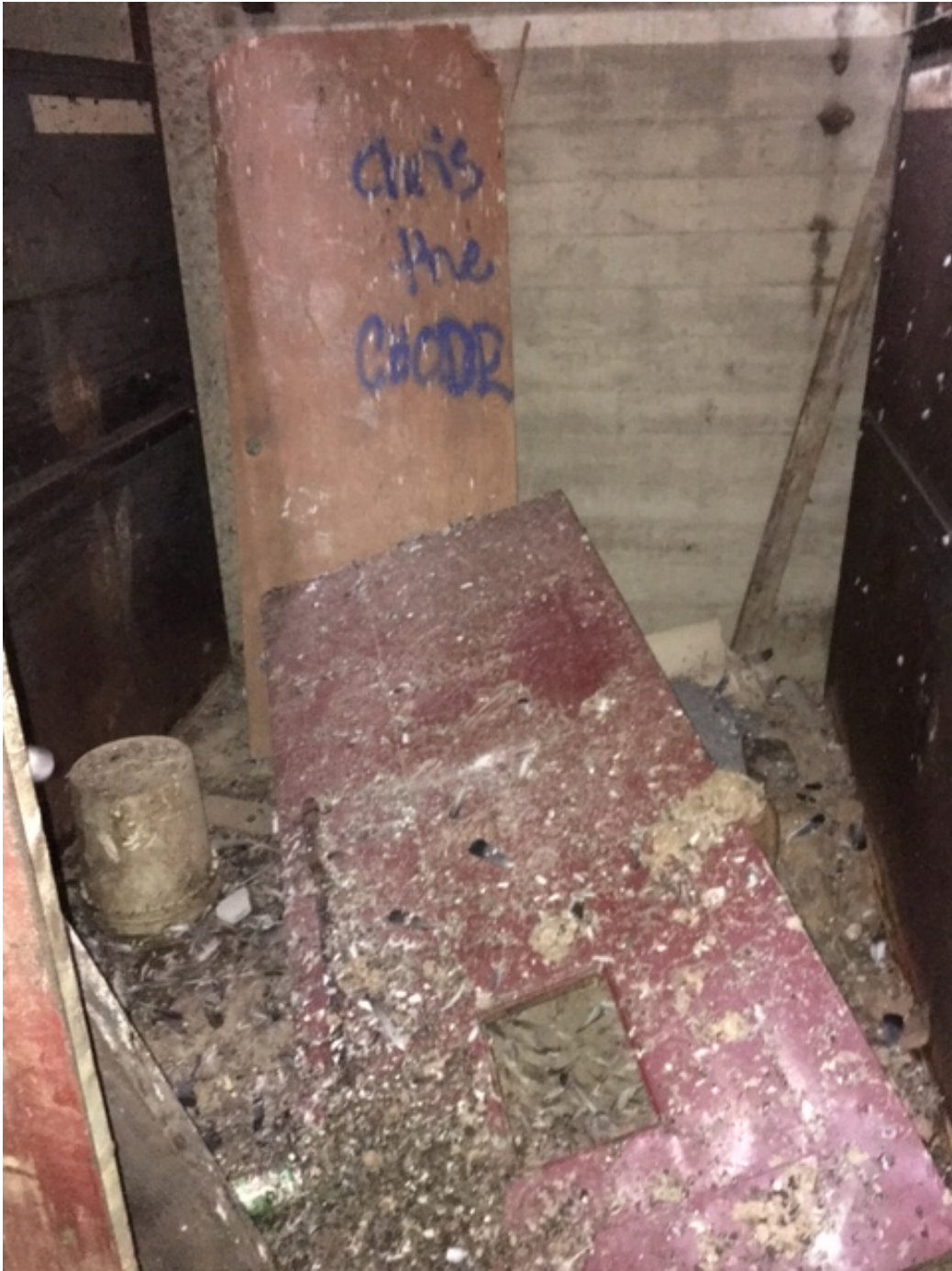
Photo 33: Debris in the elevator shaft in the basement.
