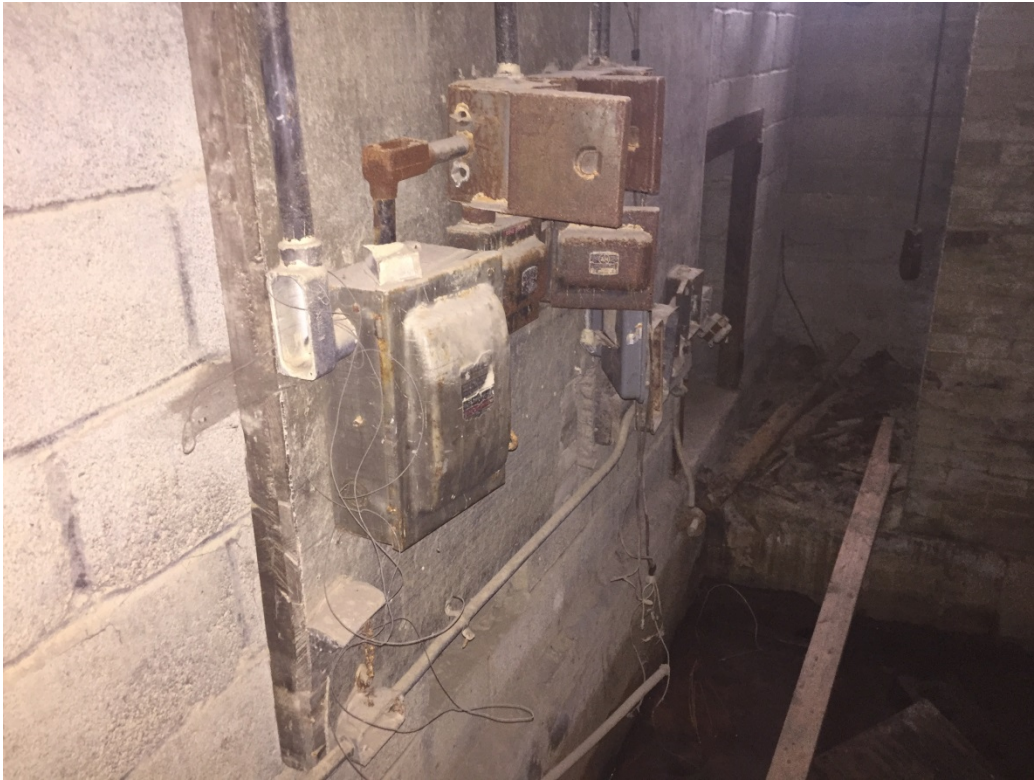
Photo 23: The electrical panel in the boiler room.
