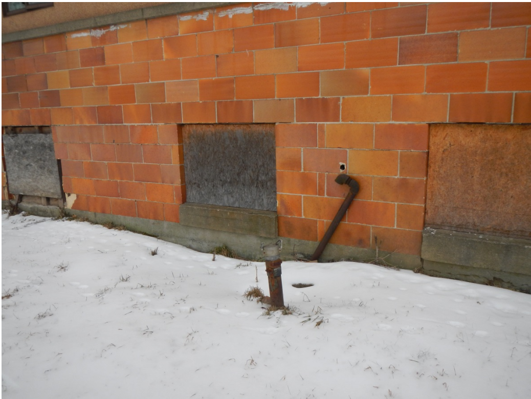
Photo 10: A fill and vent pipe located on the north wall of the building.
