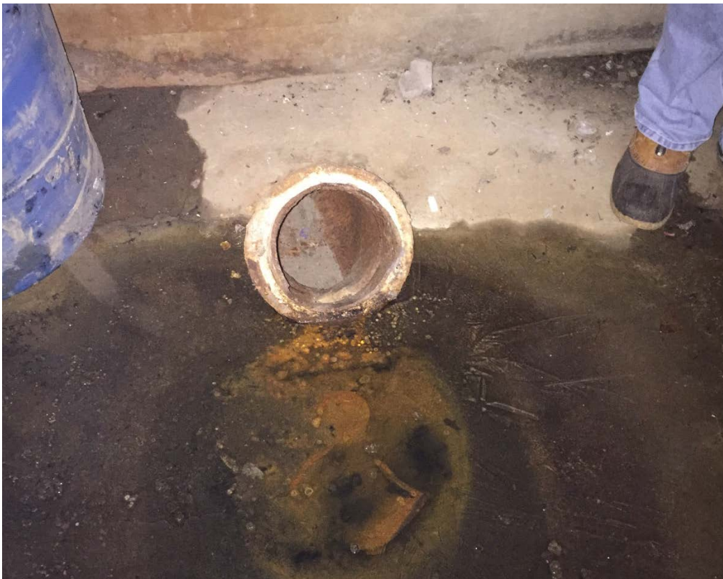
Photo 28: What appears to be a sewer clean out in the basement. A plastic 55-gallon drum can be seen next to the clean out.
