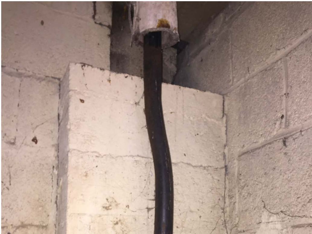
Photo 24: Suspect ACM insulation in the boiler room.
