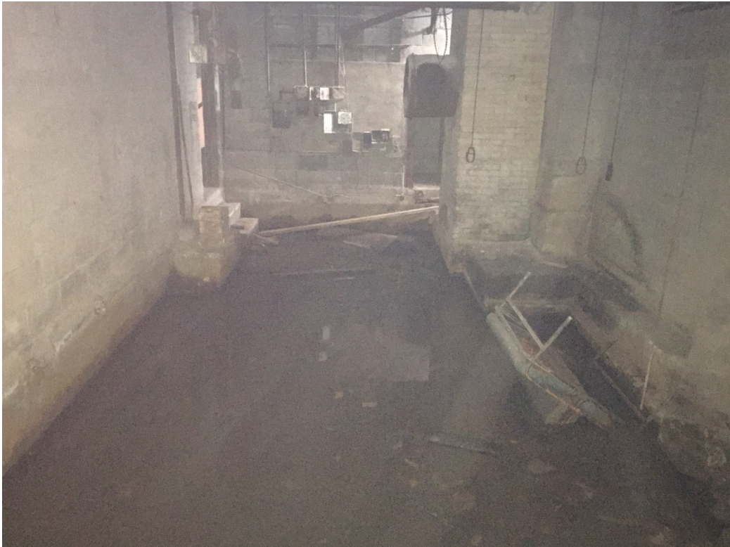
Photo 22: The boiler room in the basement east of the stairwell.
