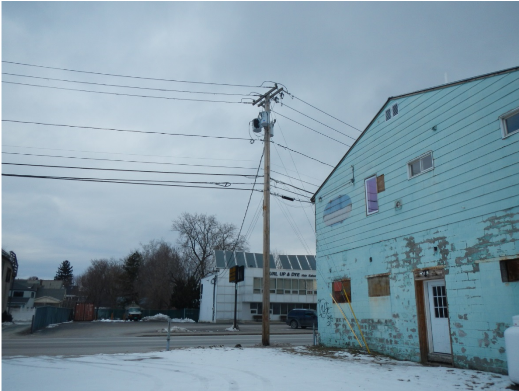
Photo 15: What appears to be a leaking transformer near the northeast property boundary. Photo taken looking northeast.
