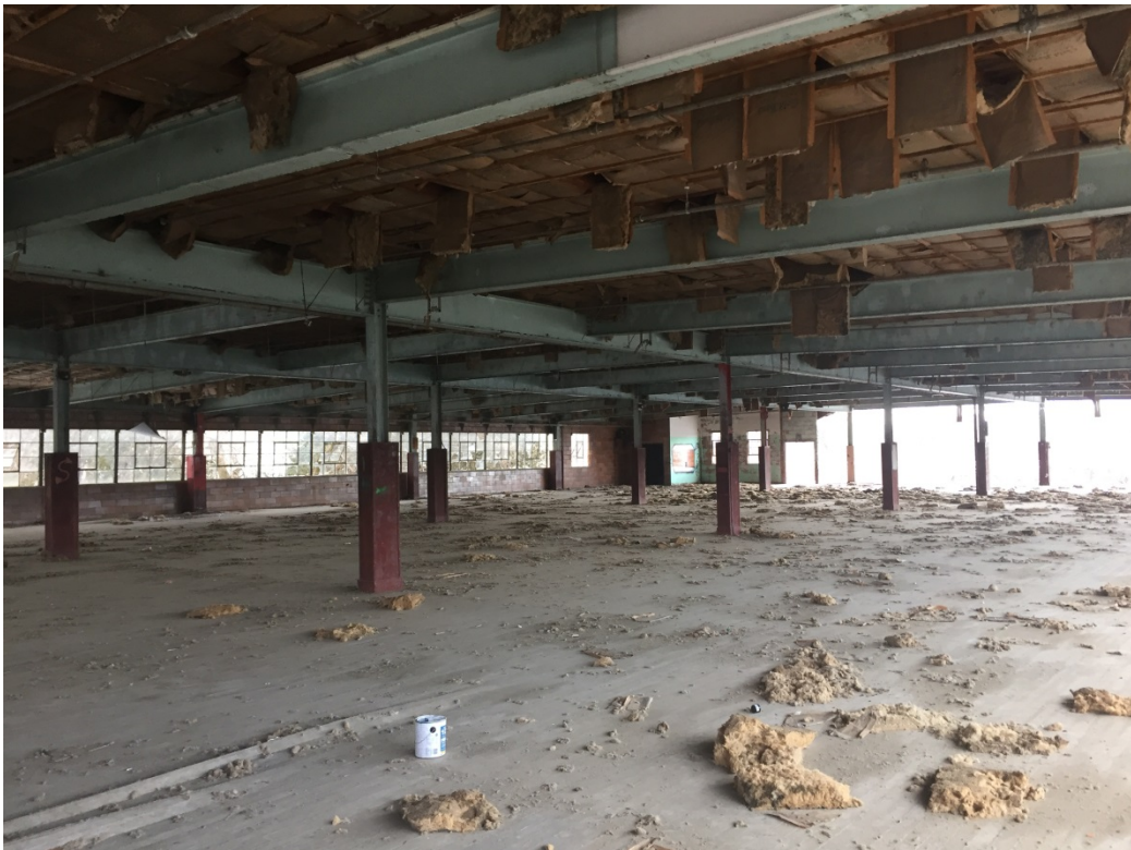
Photo 18: The top floor of the building looking southeast. The elevator shaft can be seen in the far corner of the building.
