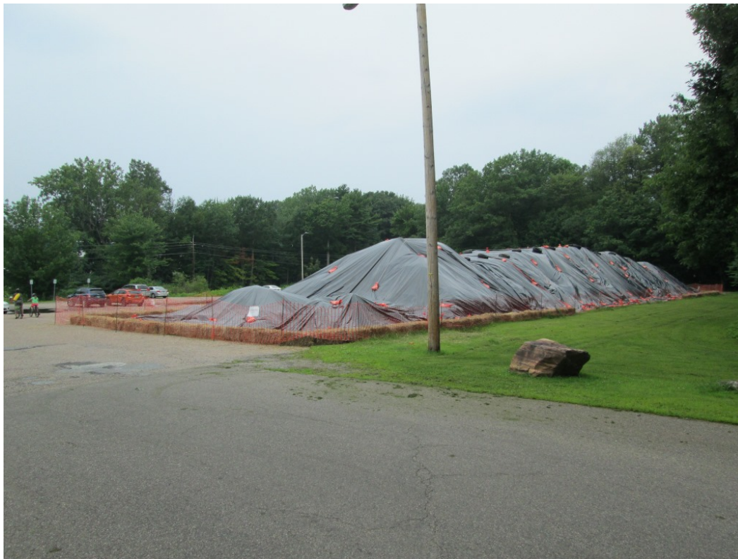
Photo 7: Soil stockpile after corrective action on 7/30/15. Photo taken looking northeast from parking lot entrance.
