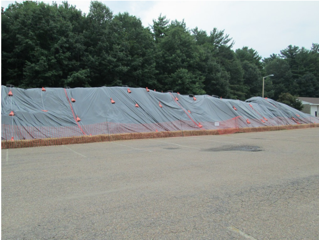
Photo 6: Soil stockpile after corrective action on 7/30/15. Photo taken looking east.
