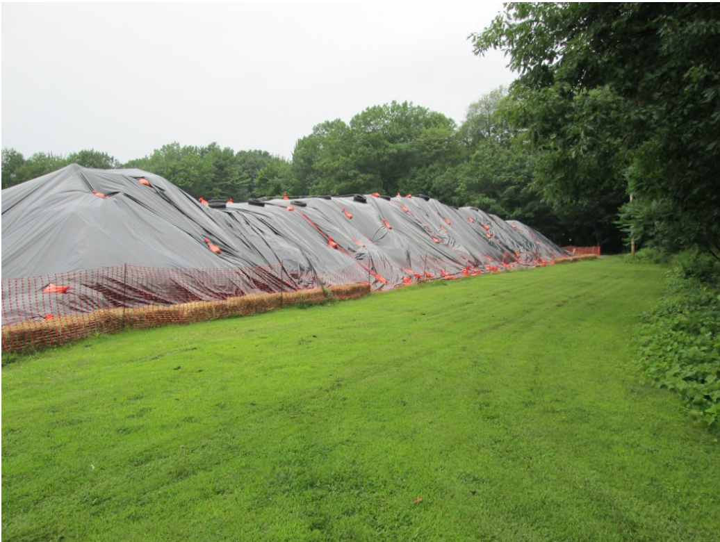
Photo 5: Soil stockpile after corrective action on 7/30/15. Photo taken looking northwest.
