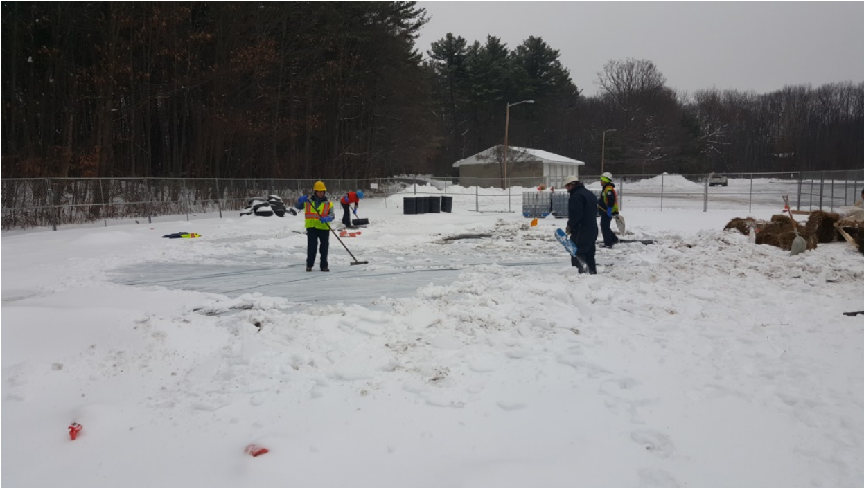
Photo 3: Shoveling snow from the poly sheeting over the final area to be cleaned.
