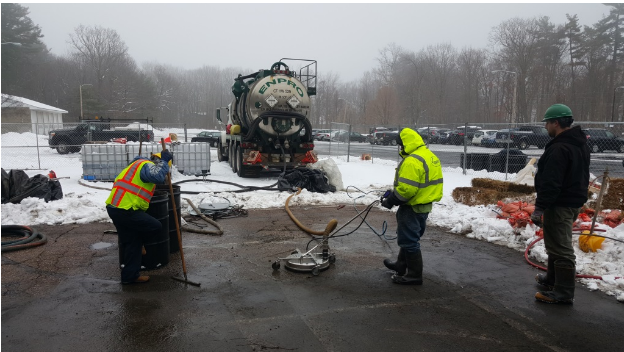
Photo 4: Cleaning the asphalt surface with the combined pressure washer and vacuum device. A rotating head sprays water onto the asphalt, loosening the dirt while the vacuum from the vacuum truck collects the wash water.
