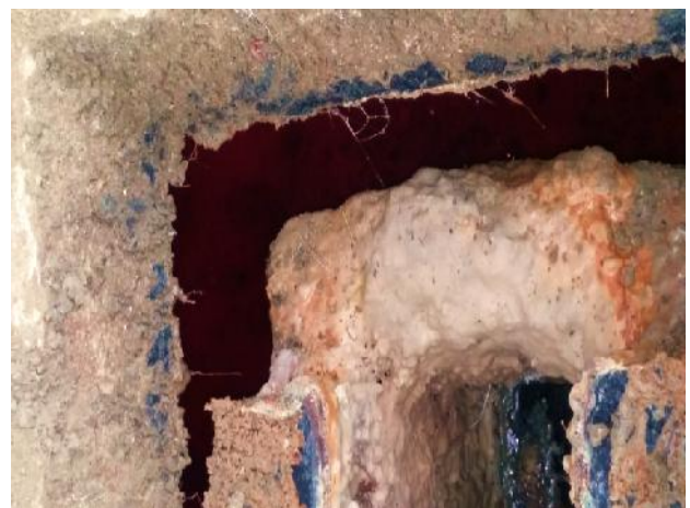
Photograph #4-Fuel Oil within Septic Tank.
