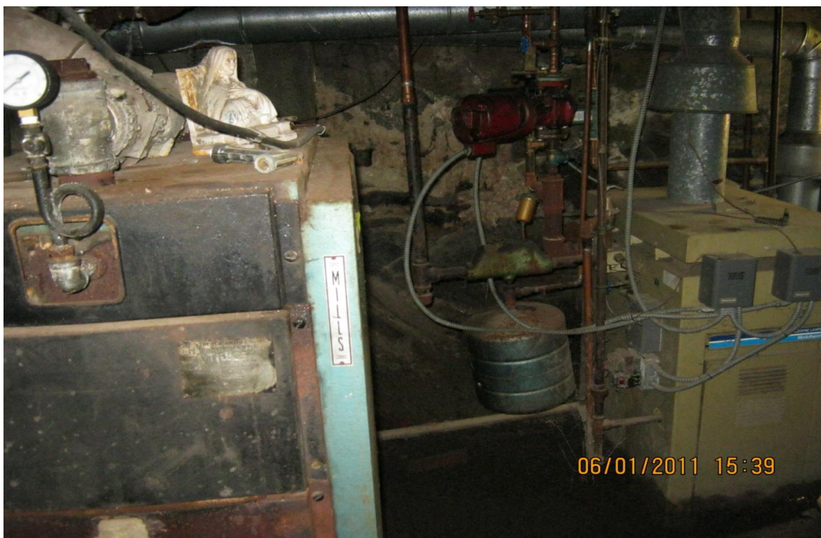
Boiler room in basement
