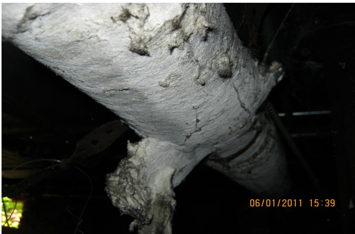
Asbestos wrapped pipe in basement
