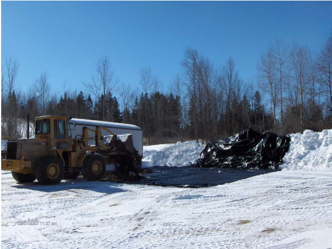
FP&H BULK STORAGE FACILITY – DERBY, VERMONT (Area of temporary Soil containment – View toward Southeast)
