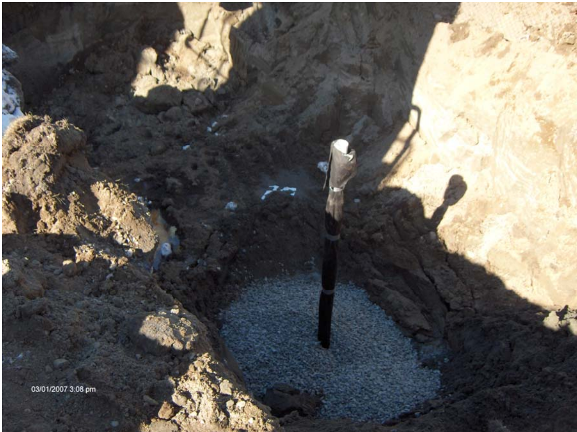
FP&H BULK STORAGE FACILITY – DERBY, VERMONT (Installation of “Excavation” Well in Berm area)
