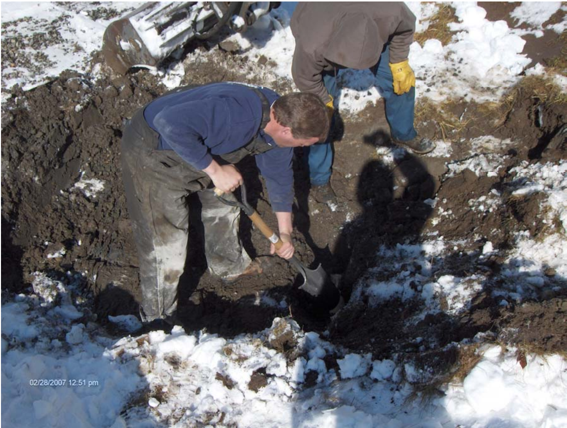
FP&H BULK STORAGE FACILITY – DERBY, VERMONT (Location of Berm drain pipe in NE corner of Berm)
