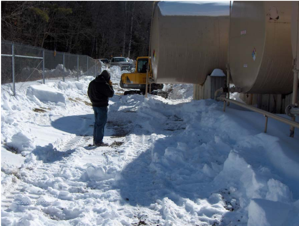
FP&H BULK STORAGE FACILITY – DERBY, VERMONT (Removal of Gas contaminated snow – View toward East)
