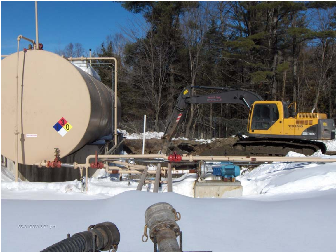
FP&H BULK STORAGE FACILITY – DERBY, VERMONT (Excavating contaminated soil in berm area – View toward North)
