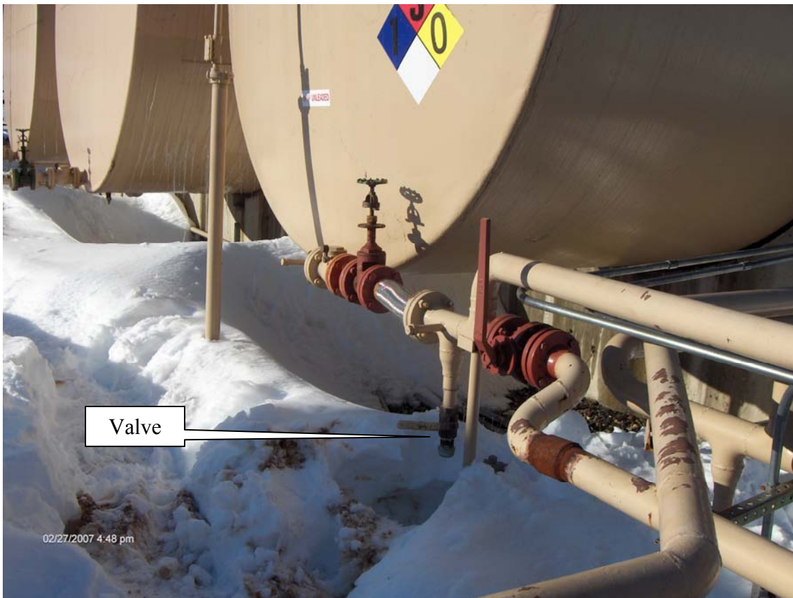
FP&H BULK STORAGE FACILITY – DERBY, VERMONT (Point of Release (Valve) – View Toward Northwest)
