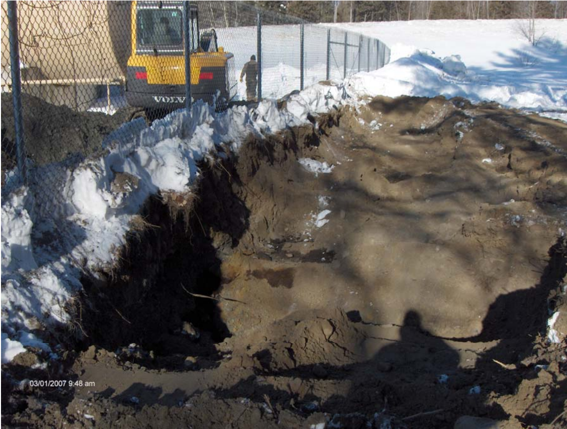
FP&H BULK STORAGE FACILITY – DERBY, VERMONT (Seepage of product during night of 28 Feb. – View Toward West-Northwest)
