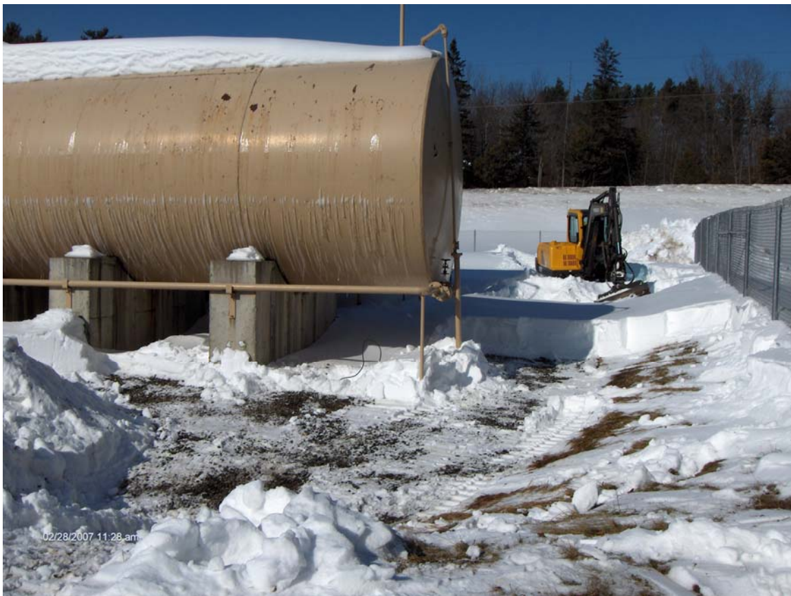
FP&H BULK STORAGE FACILITY – DERBY, VERMONT (Removal of Gas contaminated snow – View Toward West)
