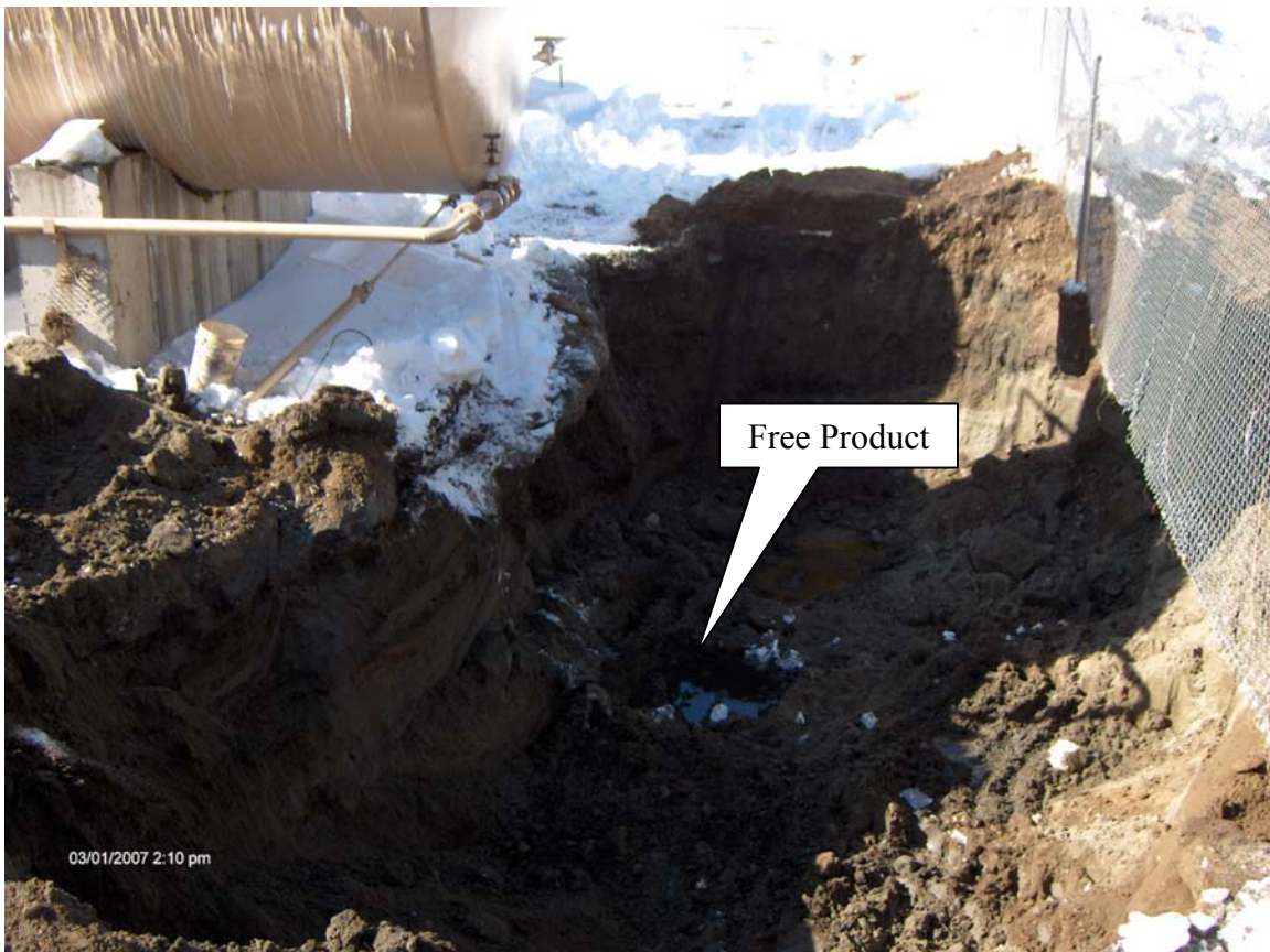
FP&H BULK STORAGE FACILITY – DERBY, VERMONT (Free product observed at 10' bgs in Berm area – View Toward West)
