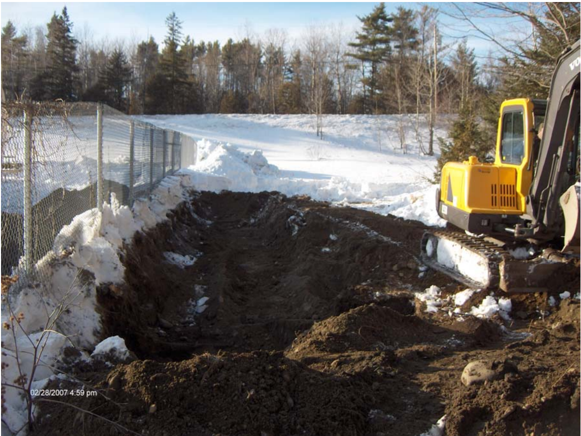
FP&H BULK STORAGE FACILITY – DERBY, VERMONT (Soil excavation to determine extent of contamination– View Toward West-Northwest)
