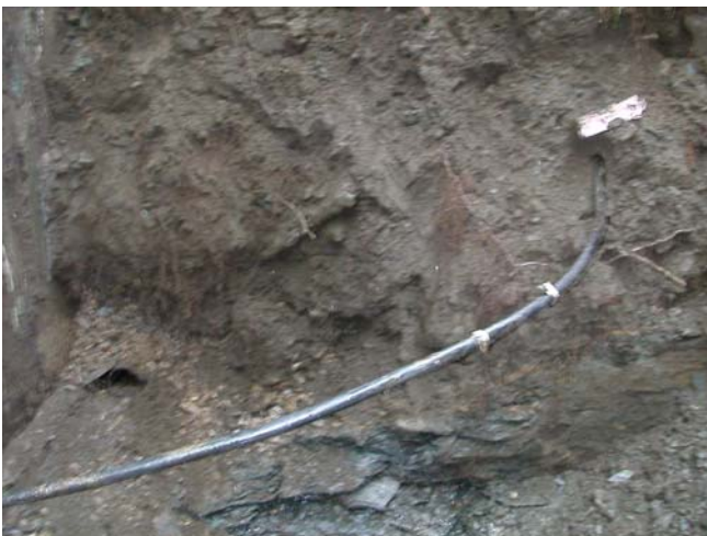
Secondary water line extending to the south from house (left). Note curtain drain along west side of house foundation. Drain was mostly filled with gravel and not considered to be a pathway for free phase oil. Note ledge immediately beneath curtain drain and house foundation.
