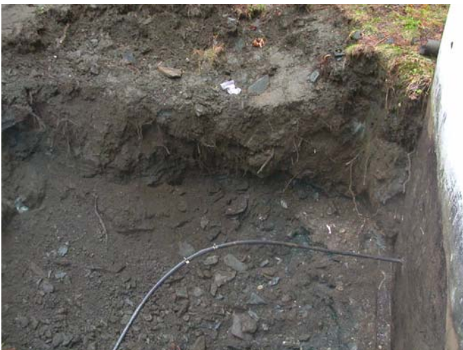
Second water line from pressure tank in basement extending south of site building. Site owner thought this line delivered water to an undetermined location, south of house. The water line from the well enters house of the north side of house, approximately 1-2 feet north of excavation pit.
