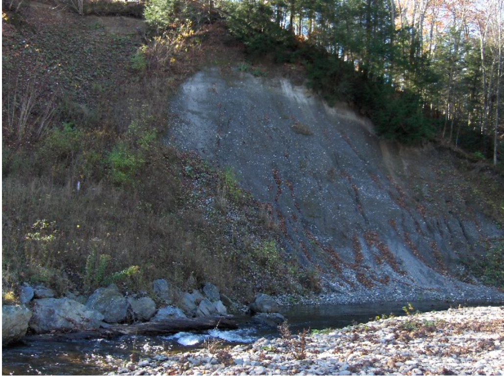
Figure 10. Mass failure on south bank of R13S3.01-C
