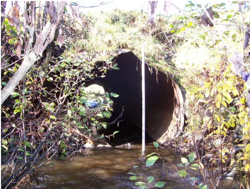
Figure 13. Brook Road culvert crossing in reach R15.07-A is undersized and impeding sediment transport. The culvert is in poor condition and has the potential to reduce AOP.
