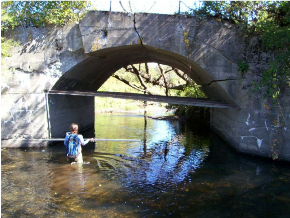
Figure 14. Farm bridge in reach R15.01-A that is structurally unsound and is causing localized geomorphic instability.
