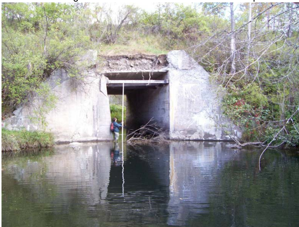
Figure 12. Rail to trail crossing in reach R15.02 has bank erosion above the outlet. This structure is undersized relative to the bankfull channel width and is recommended for replacement.
