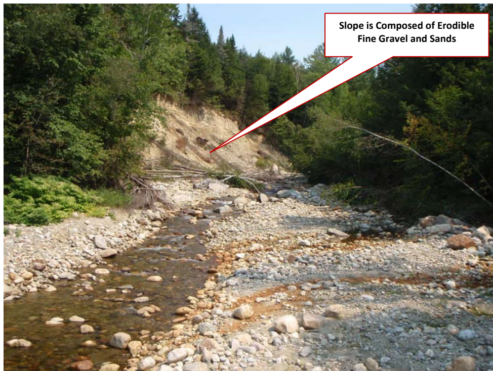
Figure 4.5 Mass failure (40' H x 330' L) located on the right (north) bank upstream of road embankment failure on Cold River Road in Shrewsbury (Segment M07-B)
