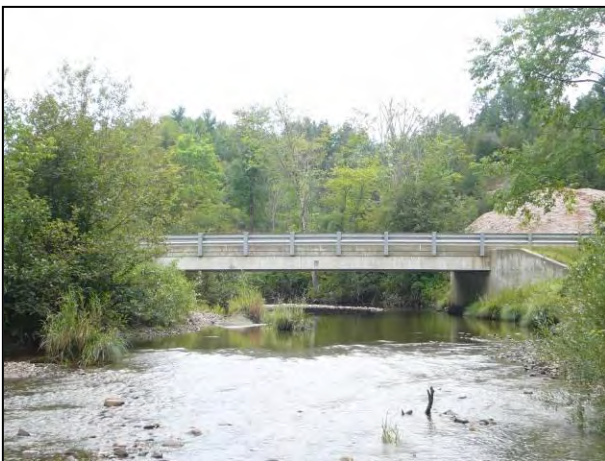
Figure 53. Undersized Route 100 bridge
