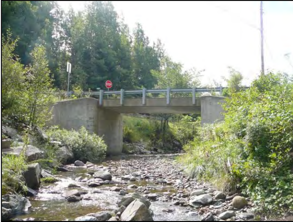
Figure 57. Undersized Rickaby Road bridge
