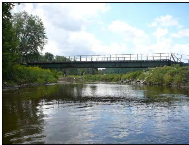
Figure 36. Undersized farm bridge
