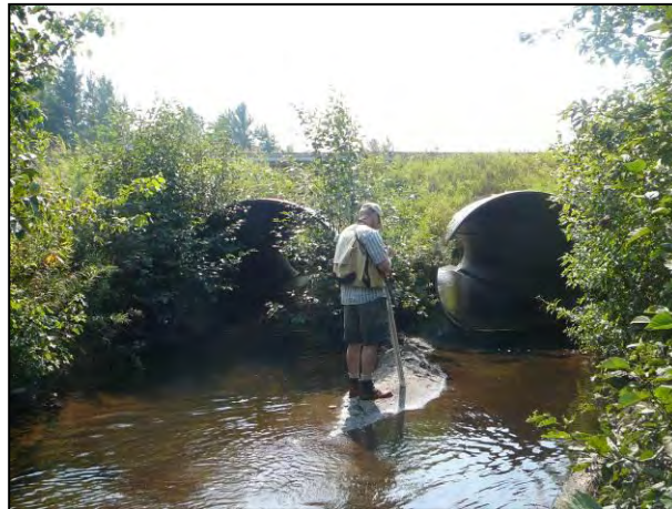
Figure 26. Undersized double culverts at Cemetery Road crossing
