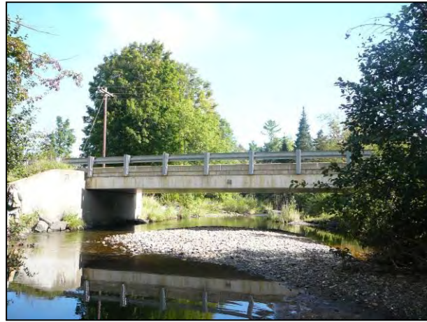
Figure 50. Undersized Lower Village Road bridge
