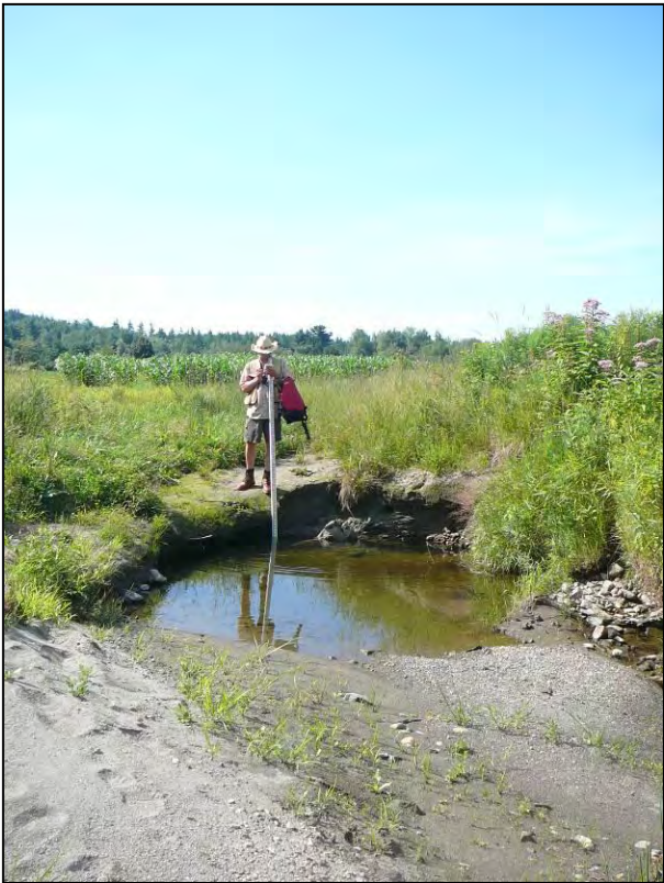
Figure 31. Active headcut on floodchute
