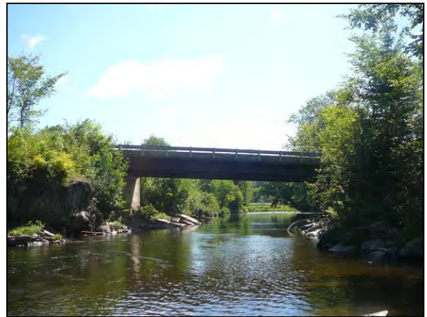
Figure 33. Undersized Loop Road Bridge
