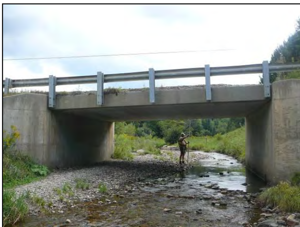
Figure 62. Undersized Cheney Road Bridge
