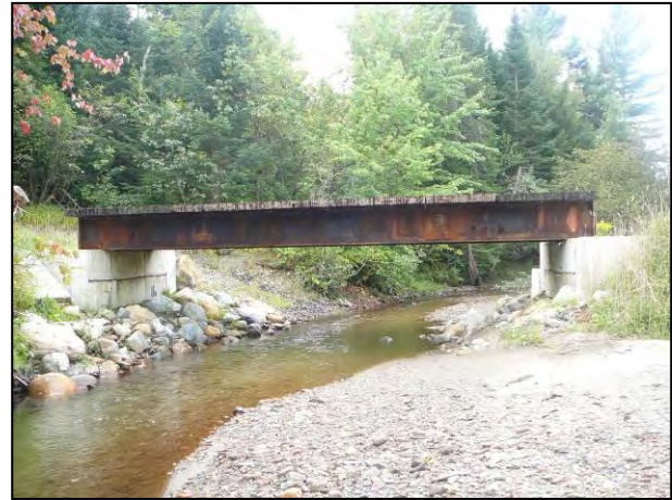
Figure 55. Undersized farm bridge
