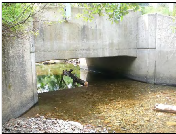
Figure 59. Undersized Private Bridge on Pierce Road
