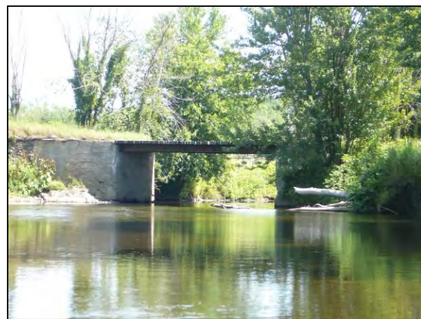
Figure 23. Undersized farm bridge
