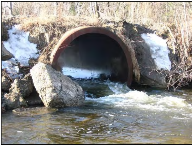
Figure 51. Undersized tube culvert
