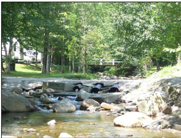
Figure 29. Undersized Triple Culverts at Campground Drive
