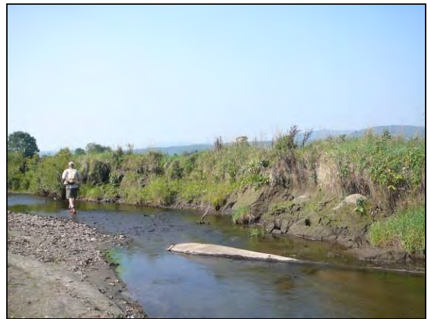
Figure 24. Erosion of outside meander bend
