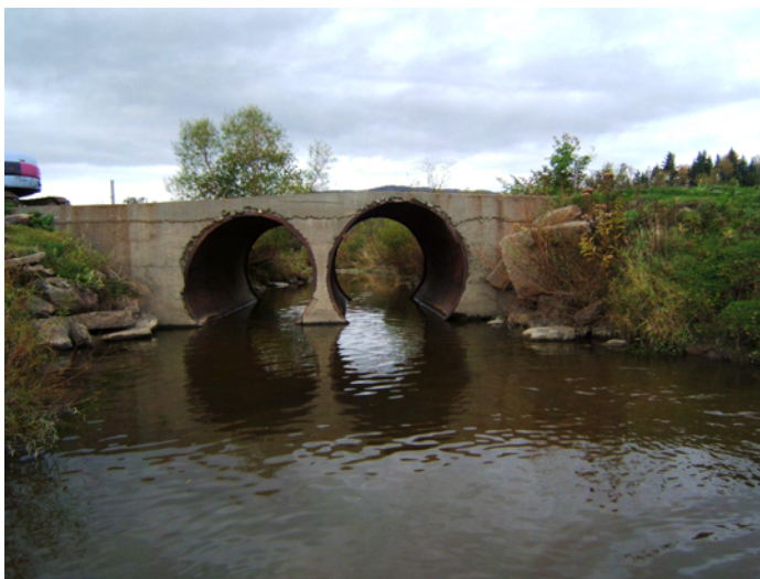
Figure xx. Segment M05A Undersized Culvert
