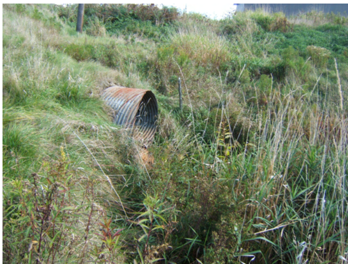
Figure rr. Rte 105 Culvert Constriction
