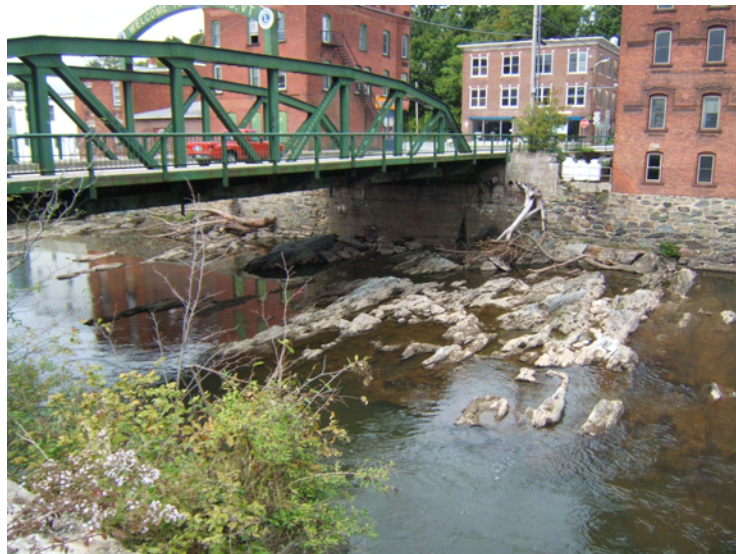
Figure i. Corridor Encroachment along Main Branch Reach R18
