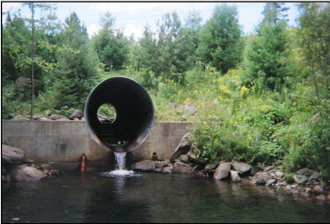
10 foot diameter culvert on Martins Brook, reach T1.04; photo taken by volunteer on 8/18/06
