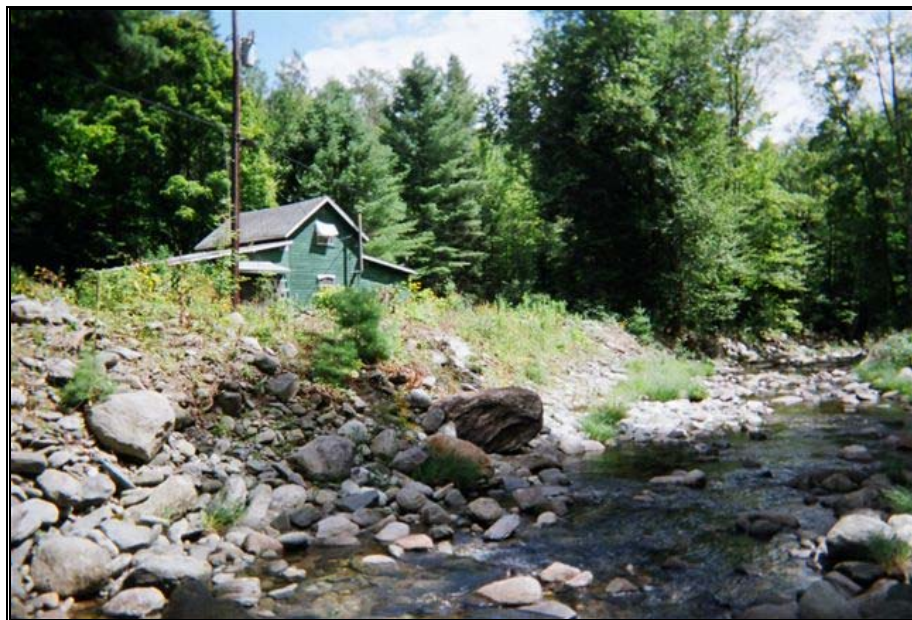
Rock rip rap bank to protect home on Martin's Brook, reach T1.03; photo taken by volunteer on 8/16/06
