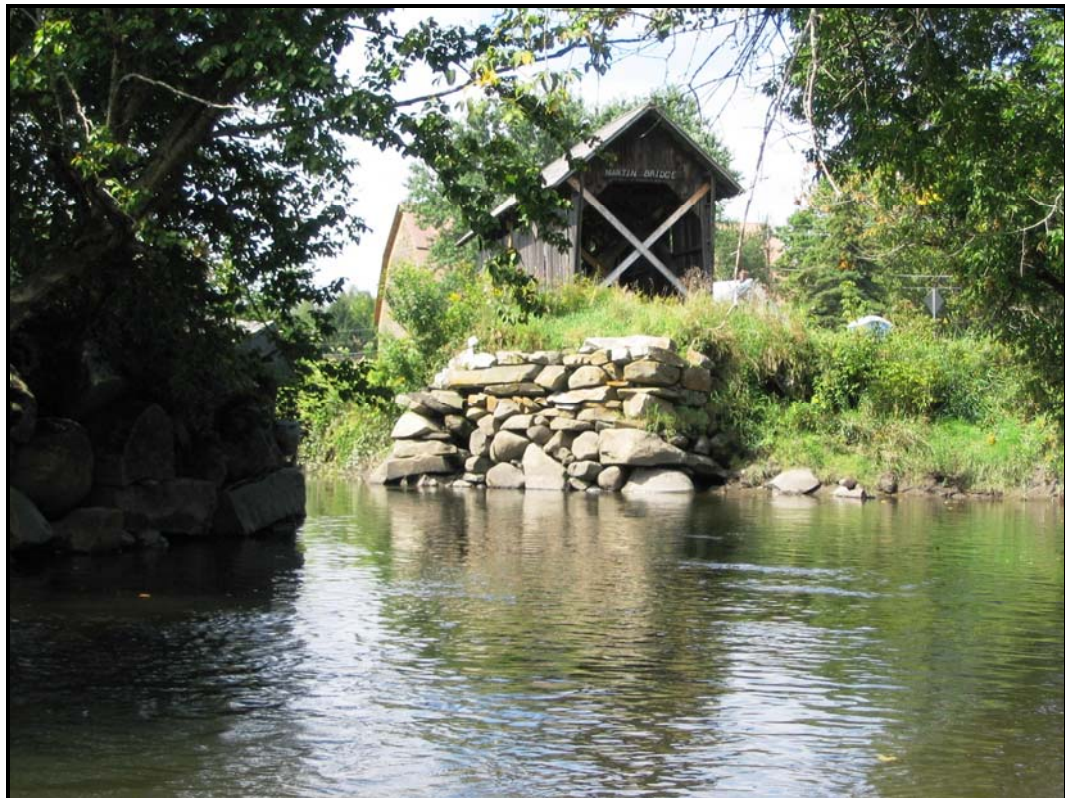
Old Bridge abutments on Reach 28 on Winooski River in Plainfield; Photo taken by TJC
