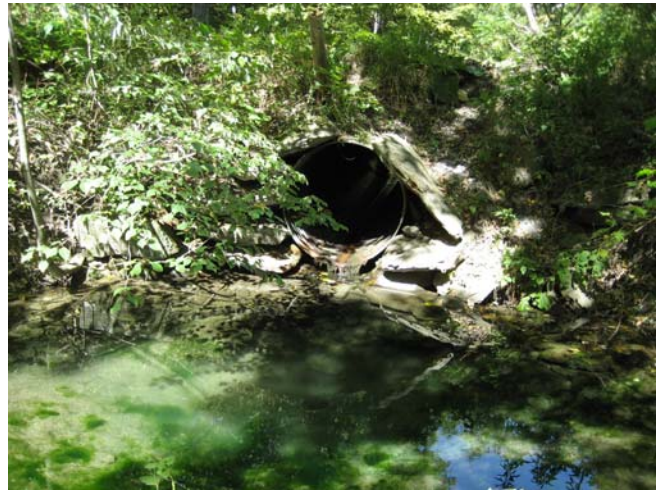
Photo 2: Downstream end of culvert under Norton Road. Deep pool sheltered many trout. Water actively flowing downstream of the culvert.
