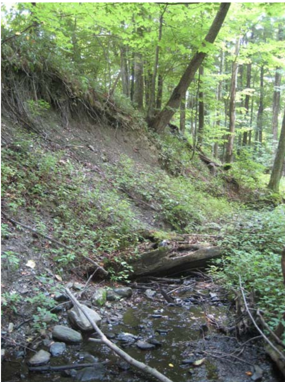
Photo 1: Erosion along valley wall. This section had lots of large woody debris.
