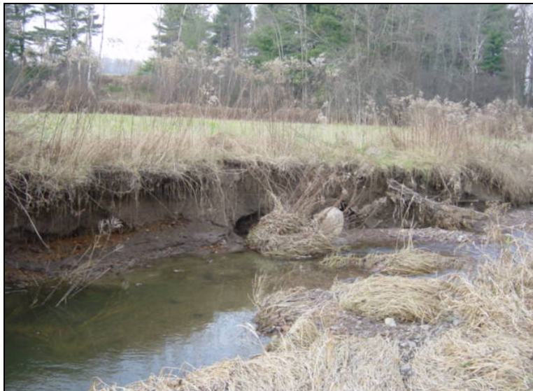
Left bank erosion with closely cropped herbaceous bank vegetation offering little bank protection.
