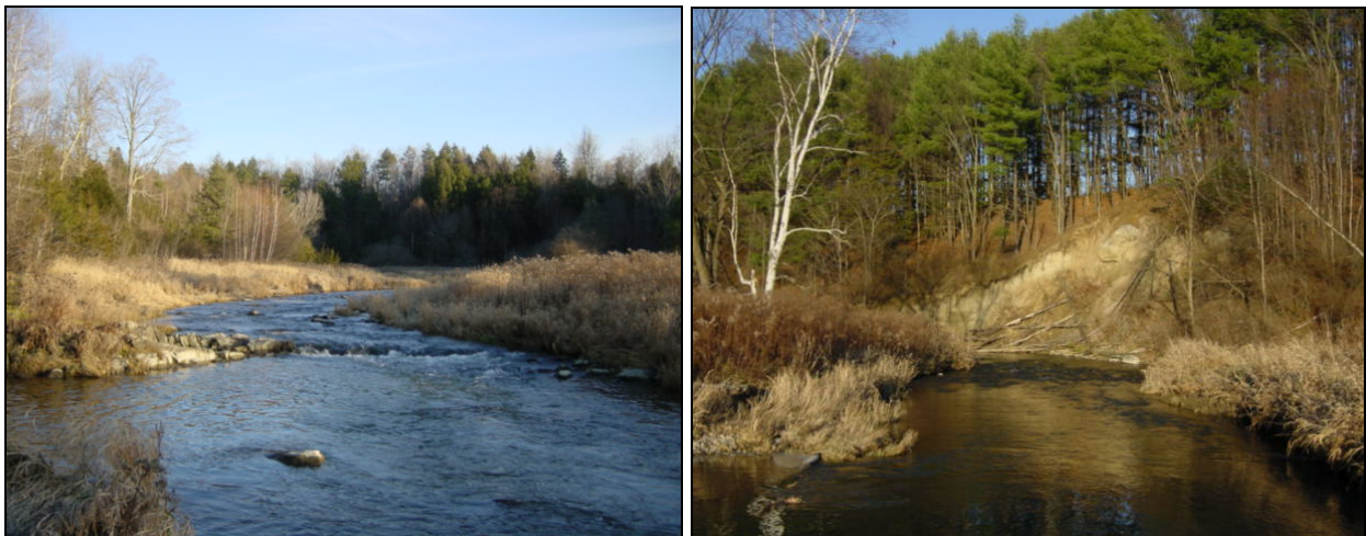
Ledge grade control and herbaceous bank vegetation (L), and one of several mass failures in the reach (R).
