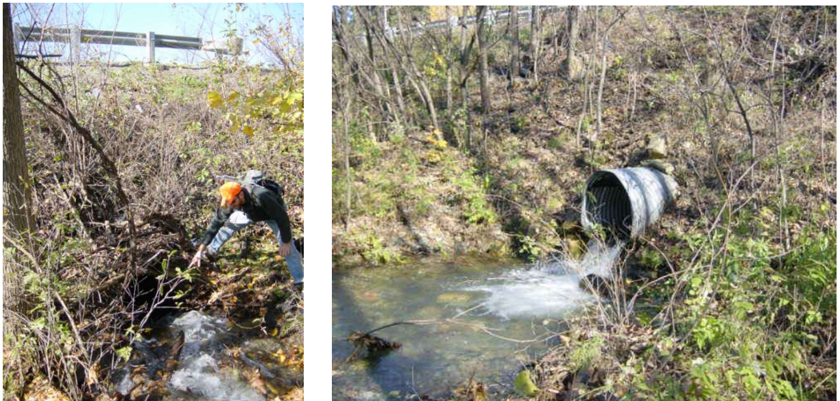
Figure 8a. Culvert on segment M18B. The upstream end of the culvert was blocked by sediment and debris and was hardly visible (left). Extreme scour was apparent at the downstream end and beyond (right).
