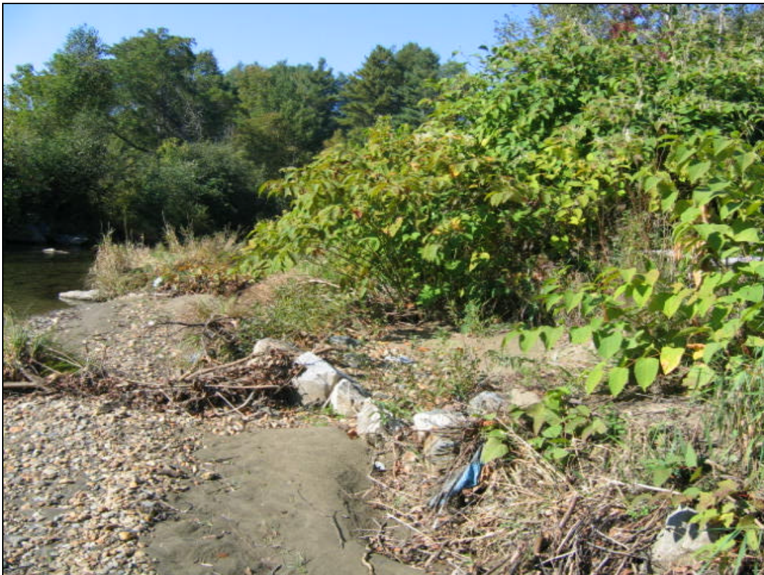
Figure 4. Planform adjustment is evident in this photograph of M3.01 where an attempt to riprap this actively moving channel had failed leaving the riprap cutting from a bar across the channel to the far bank.
