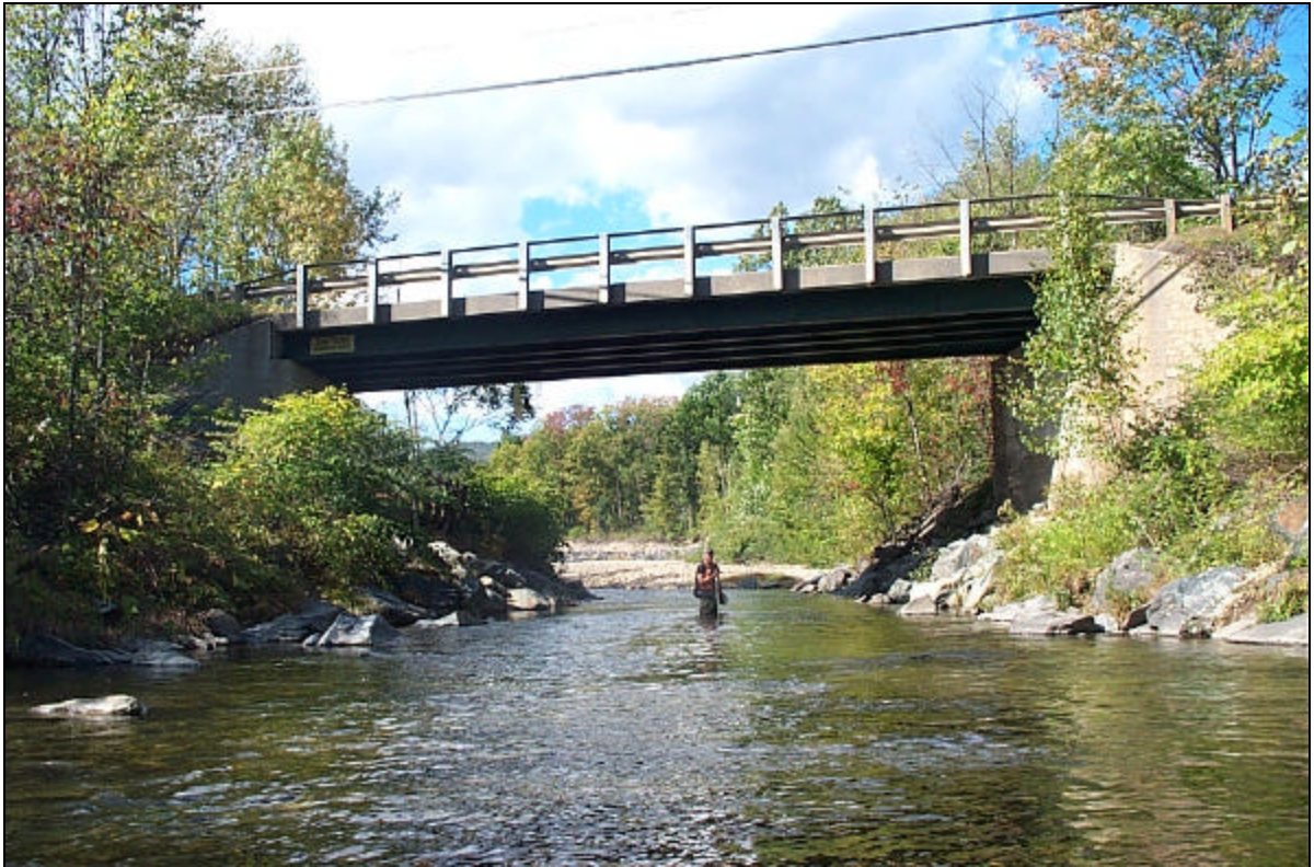
Figure 7. Luce Hill Road Bridge, a channel constriction that locally disrupts the sediment transport of the West Branch within Reach M3.02.
