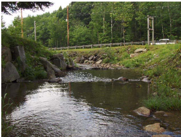
Figure 7.27. Channel alteration and armoring along Route 108 in M08.SI.01-A
