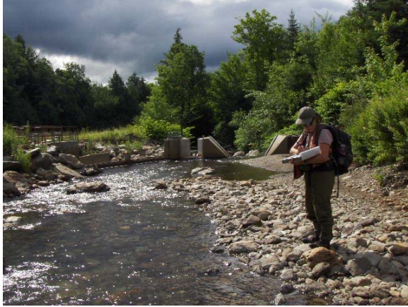
Figure 7.12. Upstream view of weir and sediment deposition in M08-C
