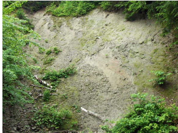
Figure 7.15. Mass failure 25 feet wide by 65 feet high along M09-A
