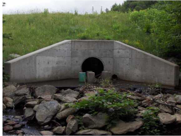
Figure 7.11. Stormwater outlet from former snowmaking pond in M08-B
