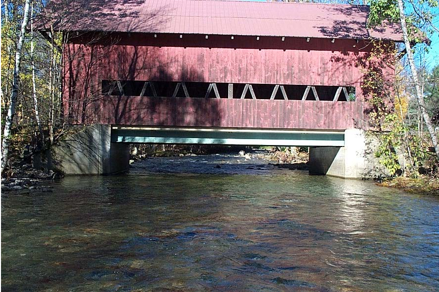
Figure 15. Undersized Brook Road Bridge
