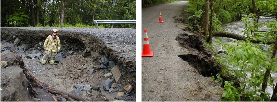
Figure 15. Sediment from portions of Gov. Mattocks Rd. taken out by South Peacham Brook suddenly became a significant contribution to stream dynamics after an intense storm in May 2011 (photos from Town of Peacham).
