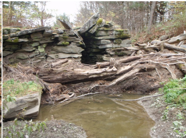
Figure 4.22 Looking downstream debris jam above the constriction
