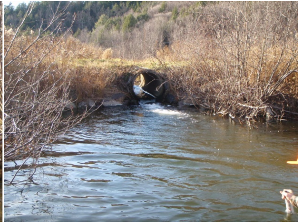
Figure 4.33 Scour-pool downstream of constricted culvert
