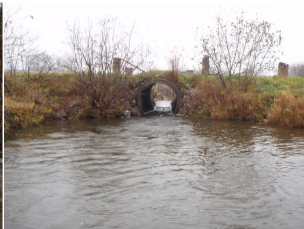
Figure 4.26 Culvert causing a large plunge pool downstream
