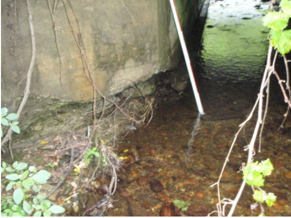
Figure 4.54 Mountain Rd crossing, with scour to the wing-walls
