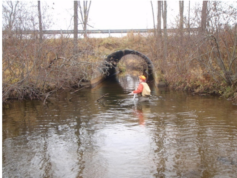
Figure 4.29 Covey Road North culvert looking upstream, some bank erosion downstream
