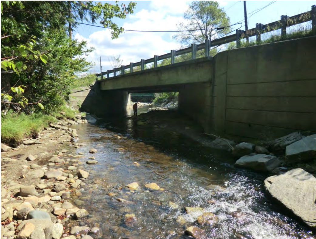
Figure 5.3. The Route 100 bridge in Dover (ID: 200013005813042) is poorly aligned and causing deposition.
