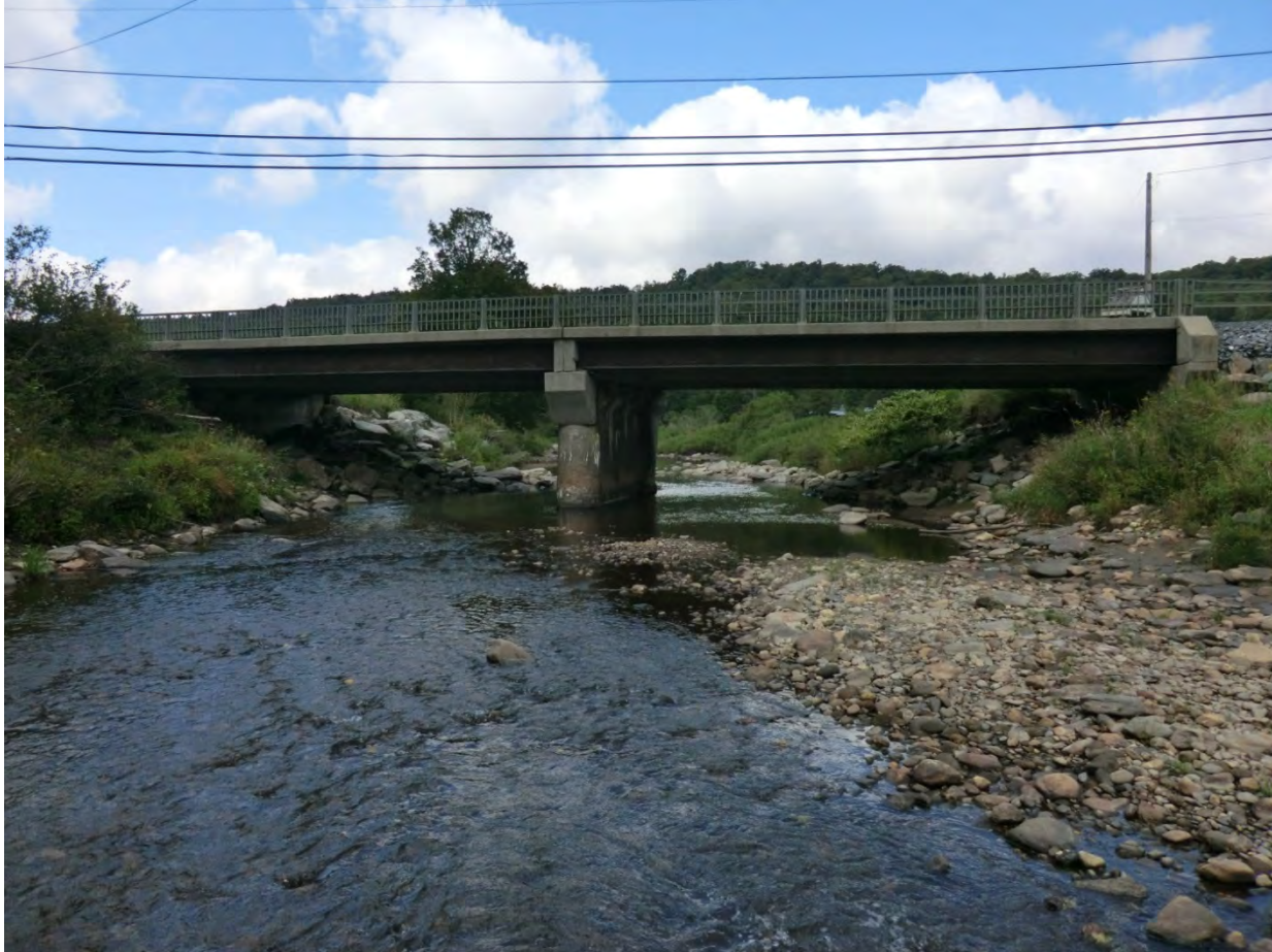
Figure 5.1. The Route 100N bridge in Wilmington is poorly aligned and is causing geomorphic instability.
