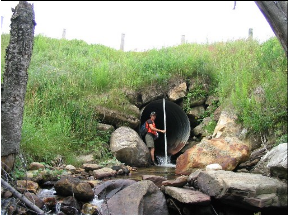
Figure 24: Undersized culverts, like this one on reach T6.08, disrupt the sediment transport capacity of the stream and often lead to both upstream and downstream destabilization.
