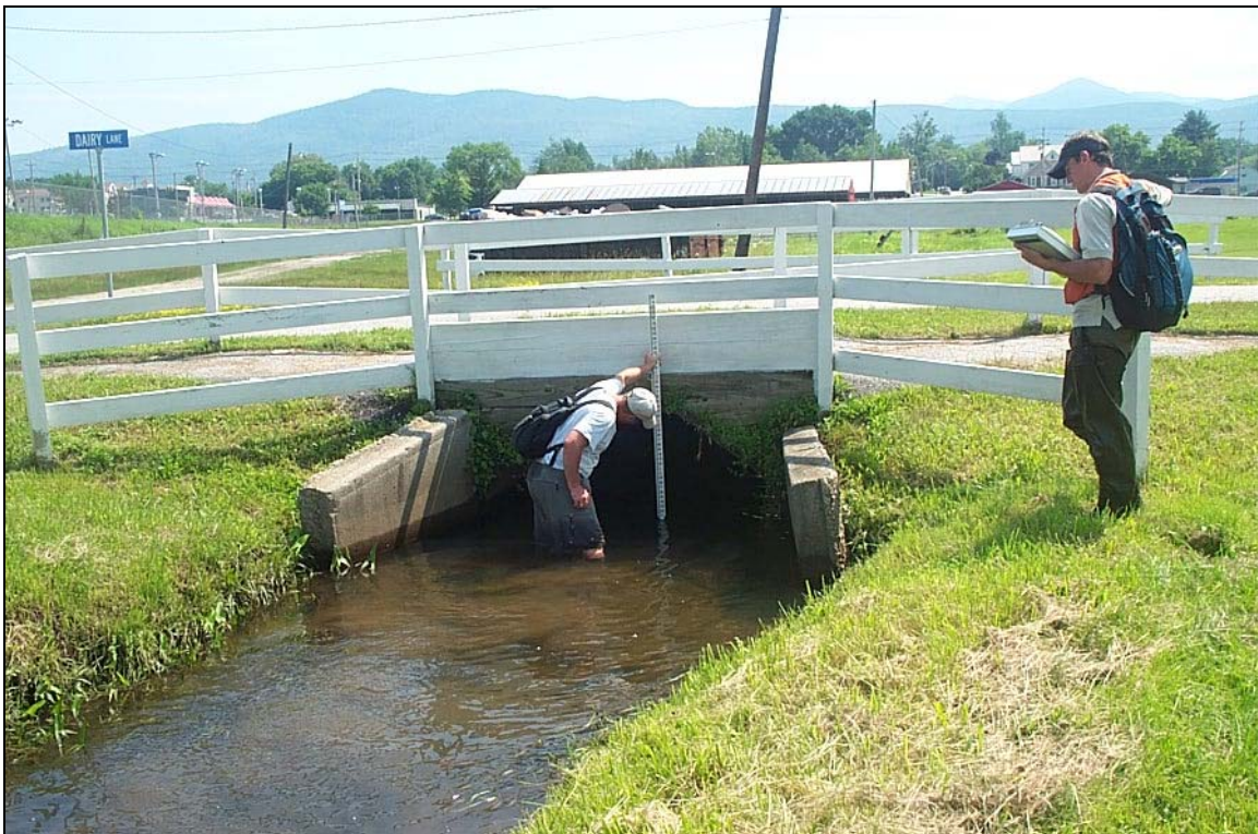
Figure 36. Undersized culverts, like this one on reach M22-S1.01-S1.01-B, disrupt the sediment transport capacity of the stream and often lead to both upstream and downstream destabilization.
