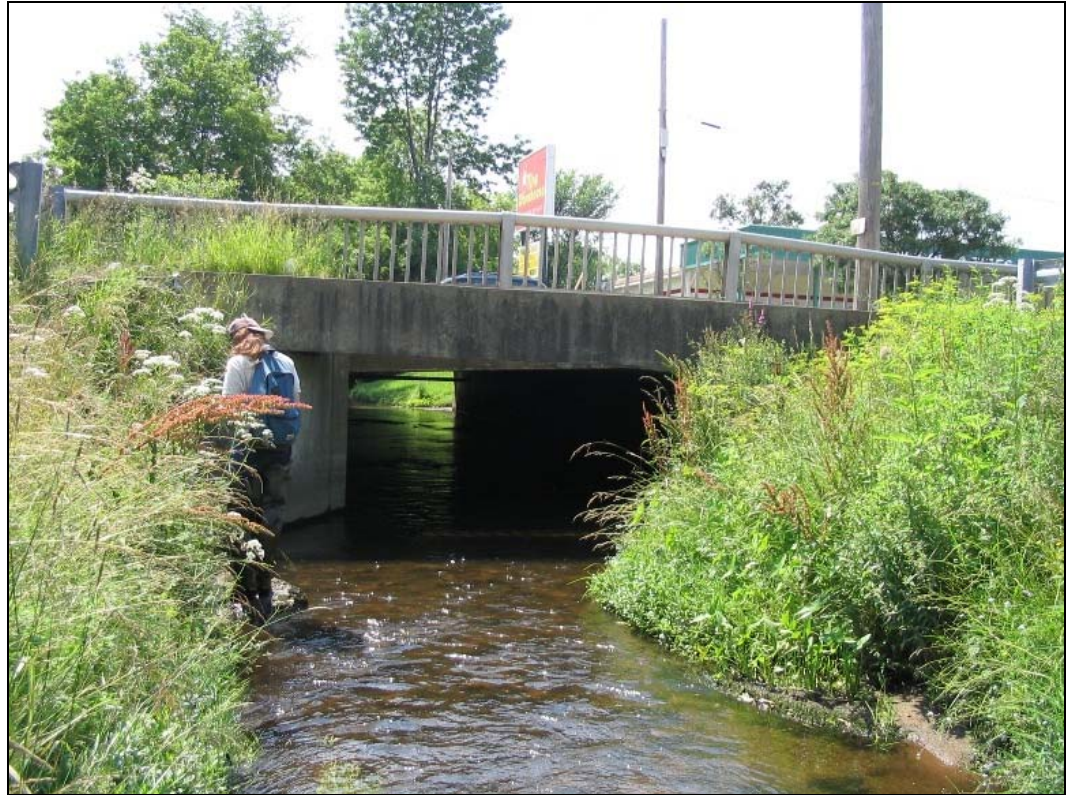
Figure I3. Segment M22-SI.02-B is heavily urbanized and has become an entrenched and extremely sensitive “G” type channel which has lost access to its historic floodplain.
