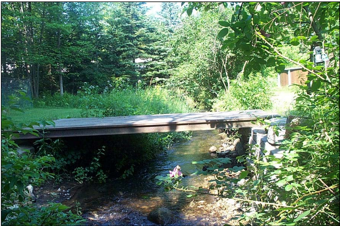
Figure 28: Segment M22-SI.01-SI.03 has been altered by floodplain encroachments and historic channel straightening. It no longer has access to a wide floodplain and has become a plane bed, “B” type stream.
