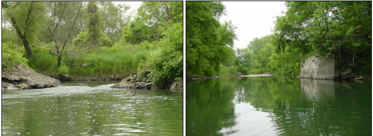
Figure 18. Old abutments constricting the channel in reach M07.
