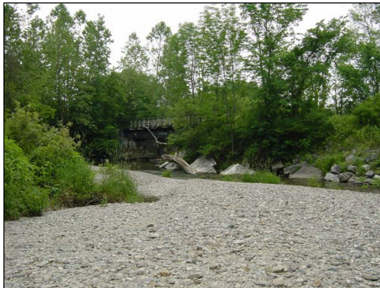
Figure 9. Bridge at the Rail Trail with heavy sediment deposits upstream.
