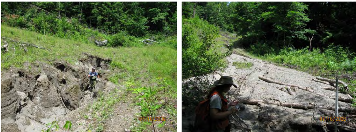
Figure 39. Gully formation (left) on logging roads in segment T1.15B resulted in significant sediment discharges to the stream (right), but large woody debris downstream and corduroy “brush bridges” still in place retained a lot of sediment and are slowing movement of these sediments. Encouragingly, the landowner and several collaborators stabilized the roads and remediated immediate impacts; follow-up visits are intended.
