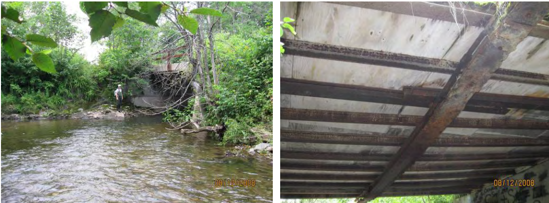
Figure 58. Bridge at Witchcat Rd. in segment T2.04B is reduced to 40% of bankfull channel width by the angle of alignment to the stream (left), appears to have possible signs of structural fatigue (right), and is recommended for further assessment regarding possible replacement.
