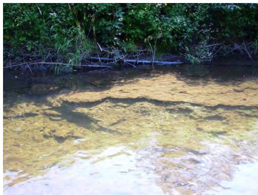
Figure 79: Beaver Meadow Brook (East Enosburgh), reach T3.01 segment B has significant left bank encroachment (upper left), bedrock grade controls (upper right). Lower segment has pond embankment that is being eroded by stream channel (bottom).
