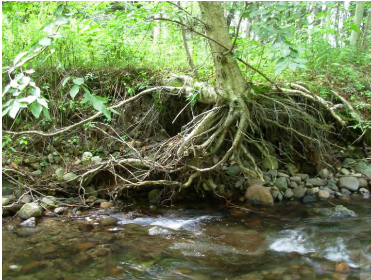
Figure 83: Reach T3S1.01 segment B has a forested buffer. Widening following incision has led to a significant amount of bank erosion and tree-fall into the stream, causing debris jams.
