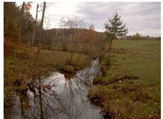
Figure 35: Reach T1.13 segment B is accessible to pastured animals, reducing buffer and causing some bank erosion.
