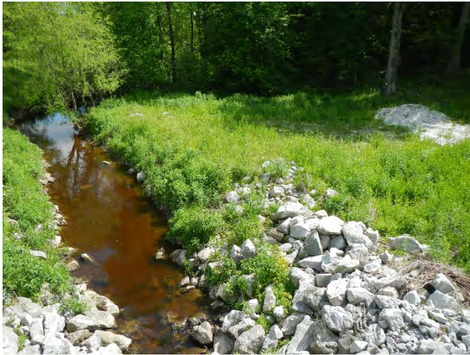
Figure 12: Bank armoring upstream of the new culvert at Chemin Pelletier S (T3.01).
