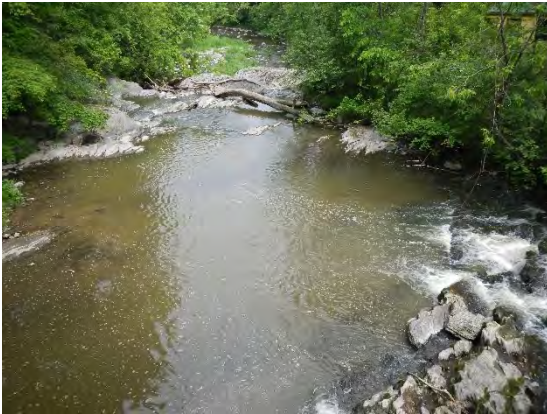
Figure 6: Start of bedrock grade control on the Rock River, north of bridge on Chemin Pelletier S.
