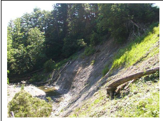
Figure 8. T3.03-B. Mass failure along right bank, mid-reach - approximately 60 feet high and 200 feet long – exposing glacial tills overlain by sandy soils.
