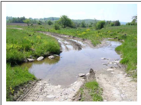
Figure 11. T3.2S1.01. View to the southeast. Active equipment ford at upstream extent of reach. Farm road providing access to this crossing also conveys stormwater runoff directly to the channel from fields to the west and northwest of the channel. Fine sediments (silts, clays, and fine sands) have accumulated in the channel coincident with the ford crossing.
