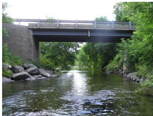
Figure 19: Hubbard Hill Bridge on Reach T202, channel constriction and associated scour
