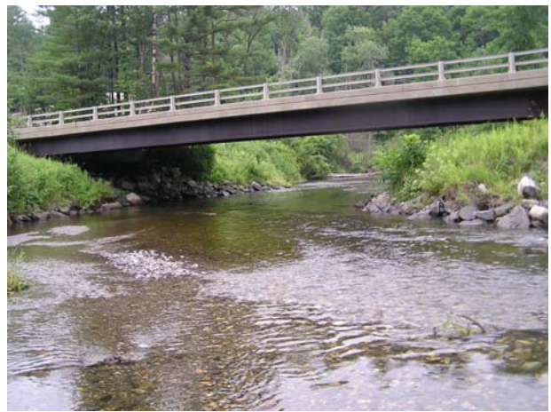
Figure 27: Photo showing Reach T204C and the upstream Bridge on Rte 122. Sediment accumulation upstream of the bridge is visible here, as well as the alignment issues of the bridge itself. While the bridge is 90' wide, riprap constricts the channel width.
