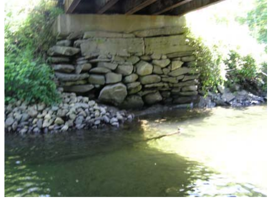
Figure 16: Farm bridge on Miller's Run Reach T201 showing potential for bridge footing failure
