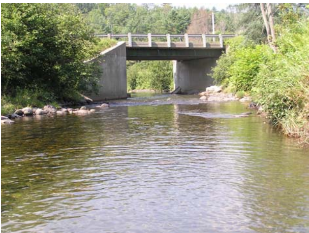
Figure 28: Photo showing the lower Rte 122 Bridge on Reach T204B. Channel upstream of the bridge is straightened the bridge is a channel constriction and long term area of conflict.
