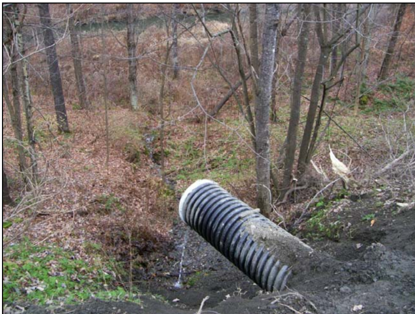
Figure 12: Road drain emptying onto steep erodable soils off of Mason Road, T2.01-C.
