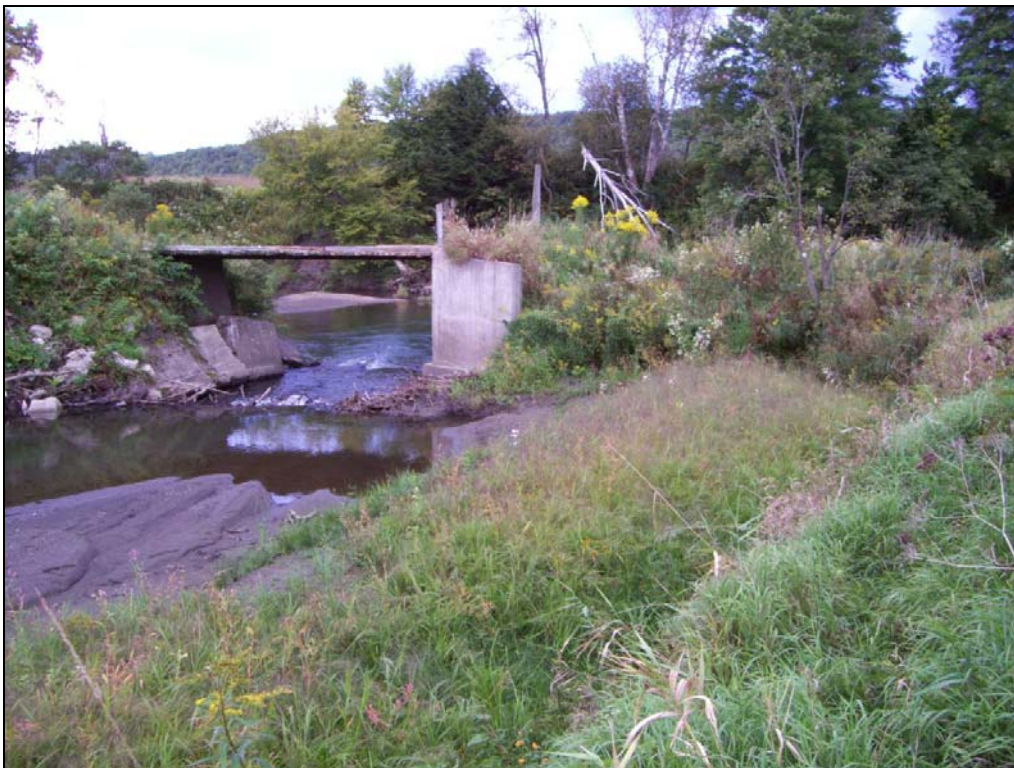
Figure 16: Example of one of many undersized structures that are significantly disrupting sediment and water transport in Ayers Brook.
