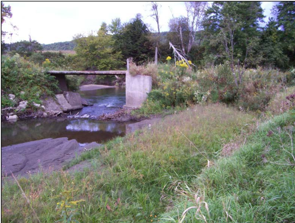
Figure 16: Example of one of many undersized structures that are significantly disrupting sediment and water transport in Ayers Brook.
