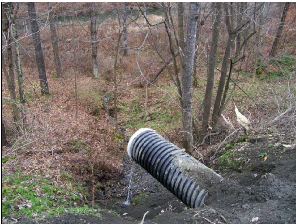
Figure 12: Road drain emptying onto steep erodible soils off of Mason Road, T2.01-C.
