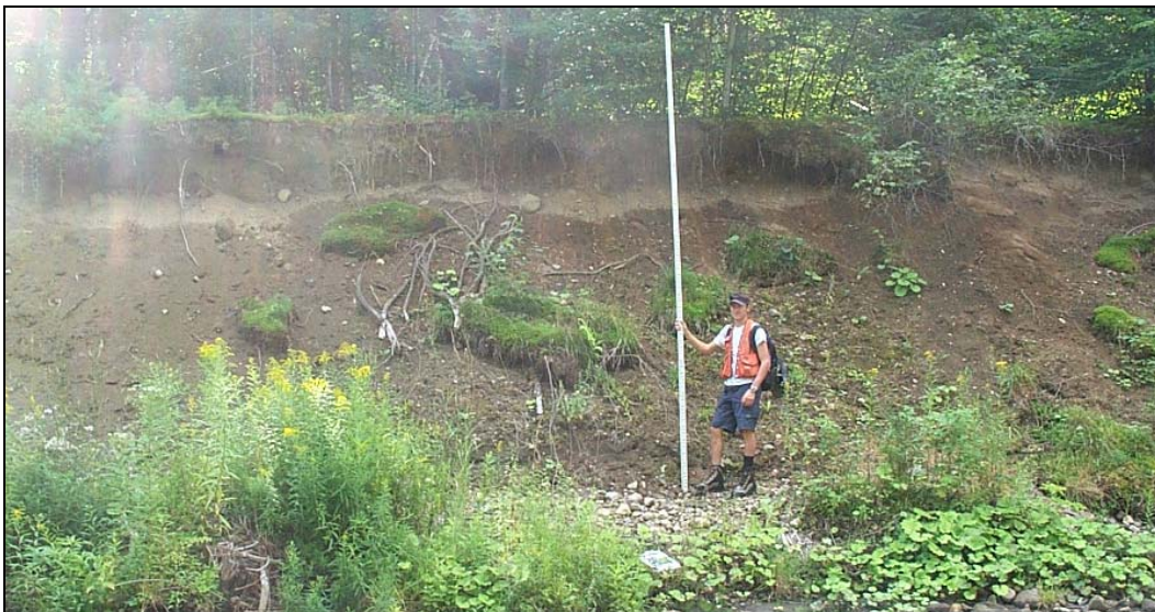
Figure 9. Massive bank failure downstream of the Tyson Road Bridge.
