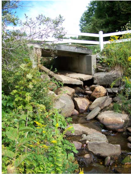
Figure 6.1 Concrete box culvert on T9.3S1.01 for a golf course path. The floor is broken and the stream flows through the cracks and emerges beneath the culvert.
