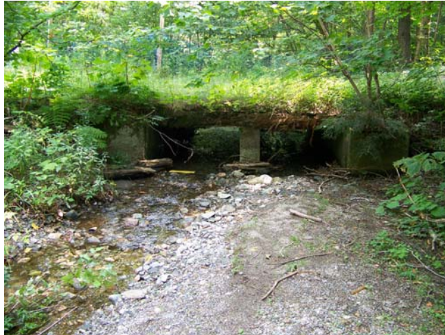
Figure 6.3 Concrete culverts on T9.3S2.01 for a path. Significant sediment has been trapped upstream and the downstream end is perched above the channel bed.
