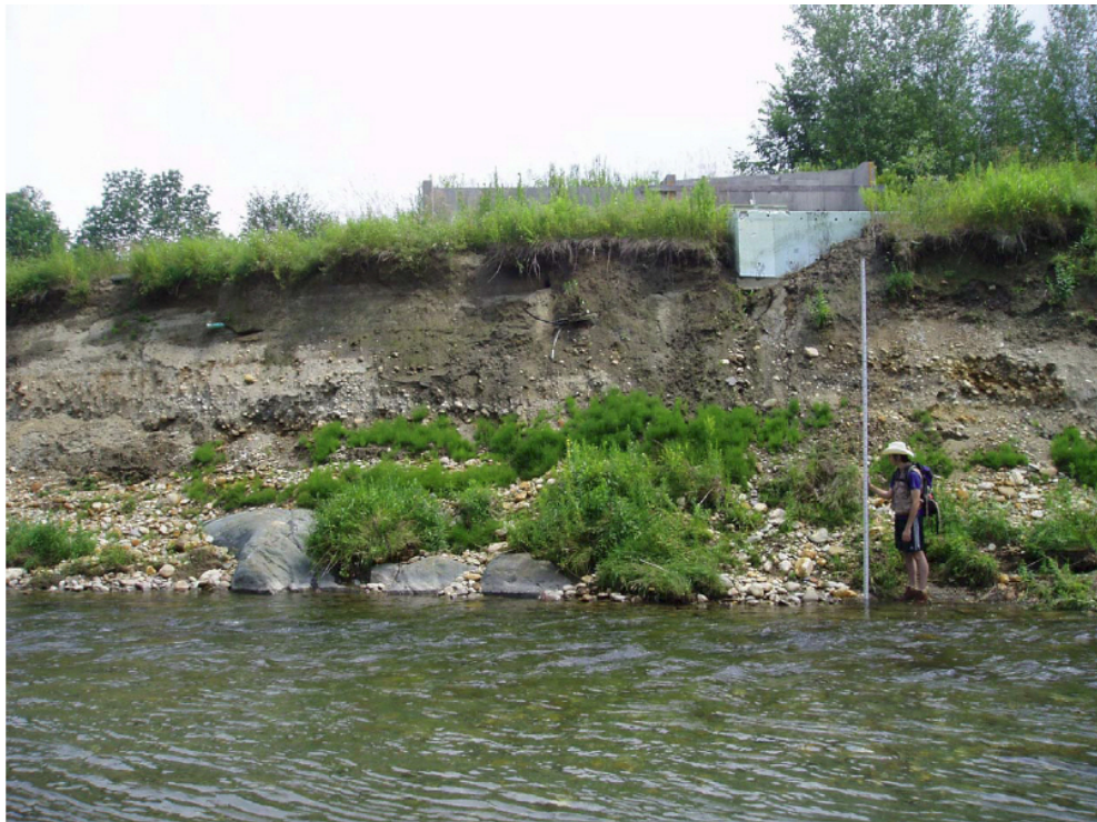
Figure 6. Eroding bank undermining foundation in Reach M15 (FGS, 2007).
